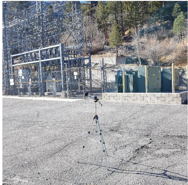
Northeast of Tailrace Near Electrical Switching Station
