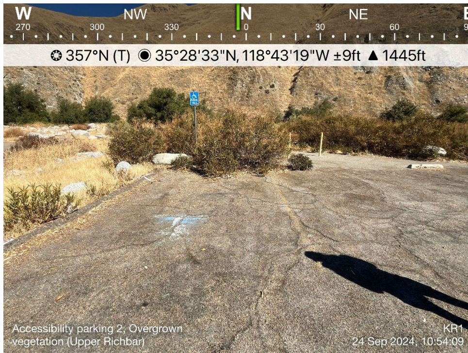
Photo B-27. Upper Richbar Day Use Site – East Parking Lot and ADA Parking Spots
