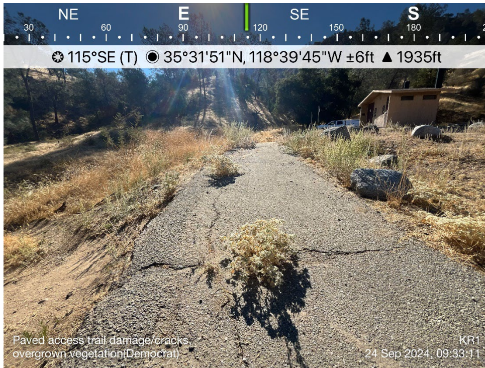
Photo B-12. Democrat Raft Take-out Boating Site – Paved Access Path and Overgrown Vegetation
