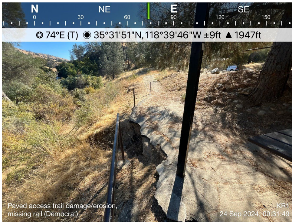
Photo B-13. Democrat Raft Take-out Boating Site – Paved Access Trail with Missing Handrails, Erosion and Wash Out
