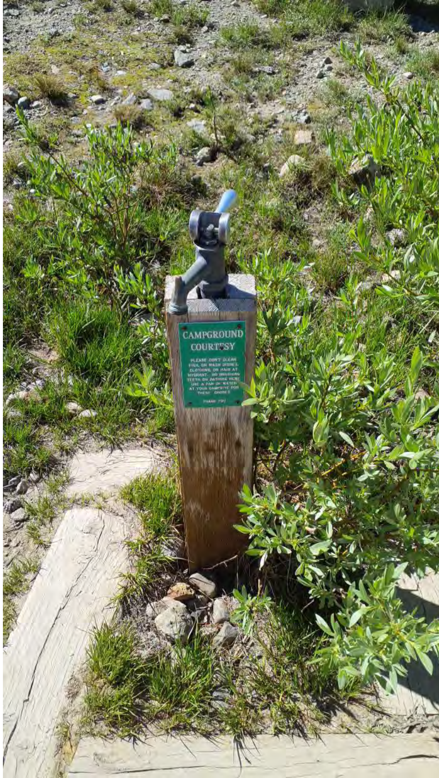
Photo 15. Saddlebag Lake Day Use Area, Potable Water Pump
