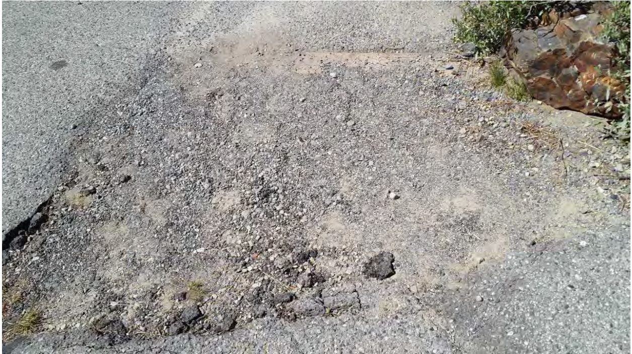
Photo 47. Ellery Lake Campground, Erosion
