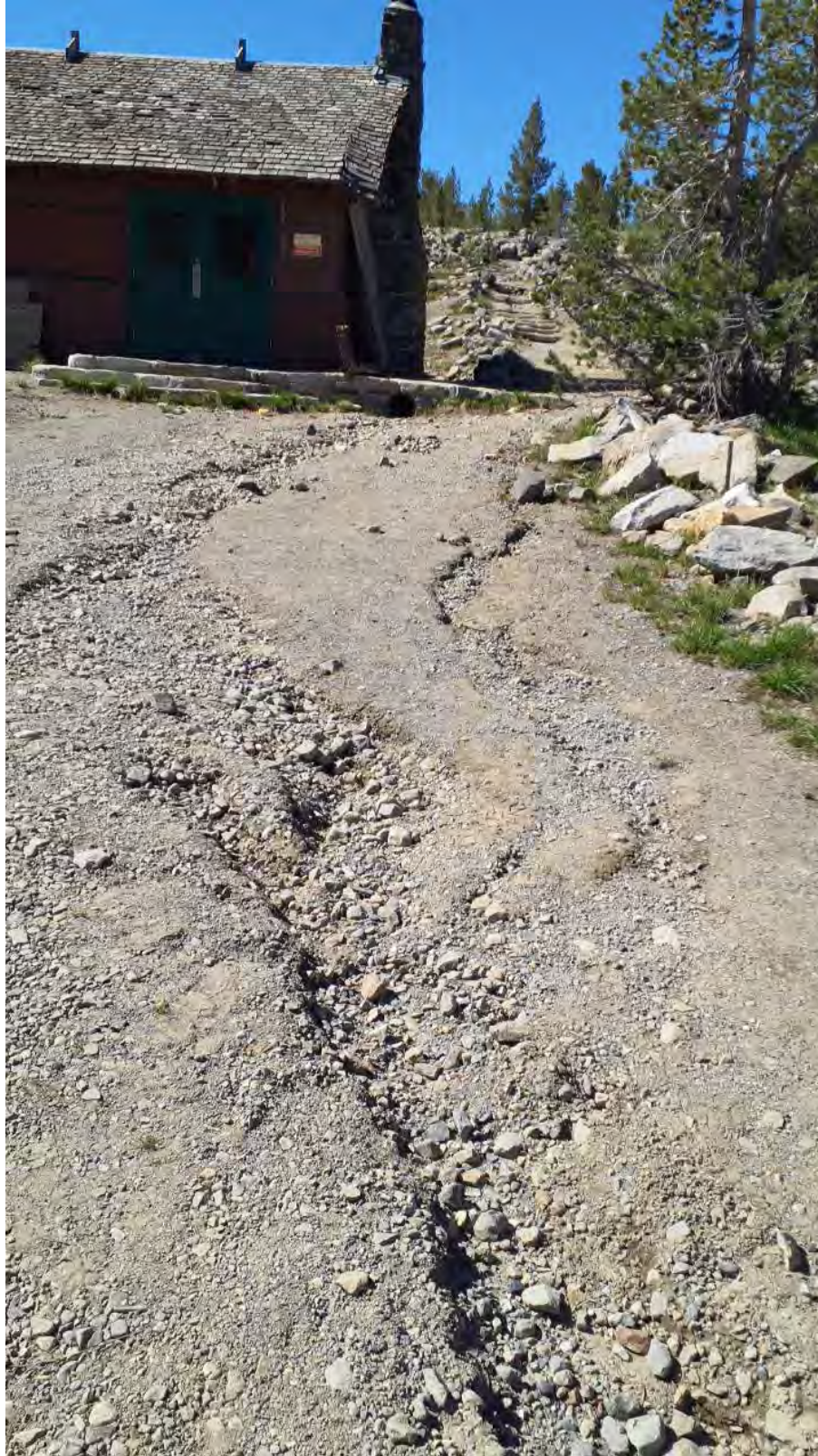
Photo 19. Saddlebag Lake Day Use Area, Erosion
