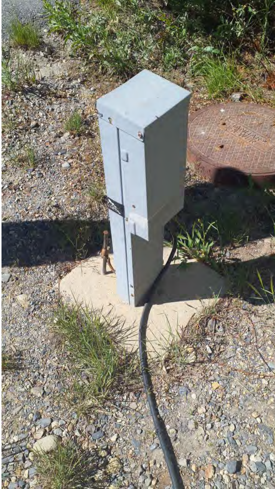
Photo 50. Ellery Lake Campground, Electrical Hookup
