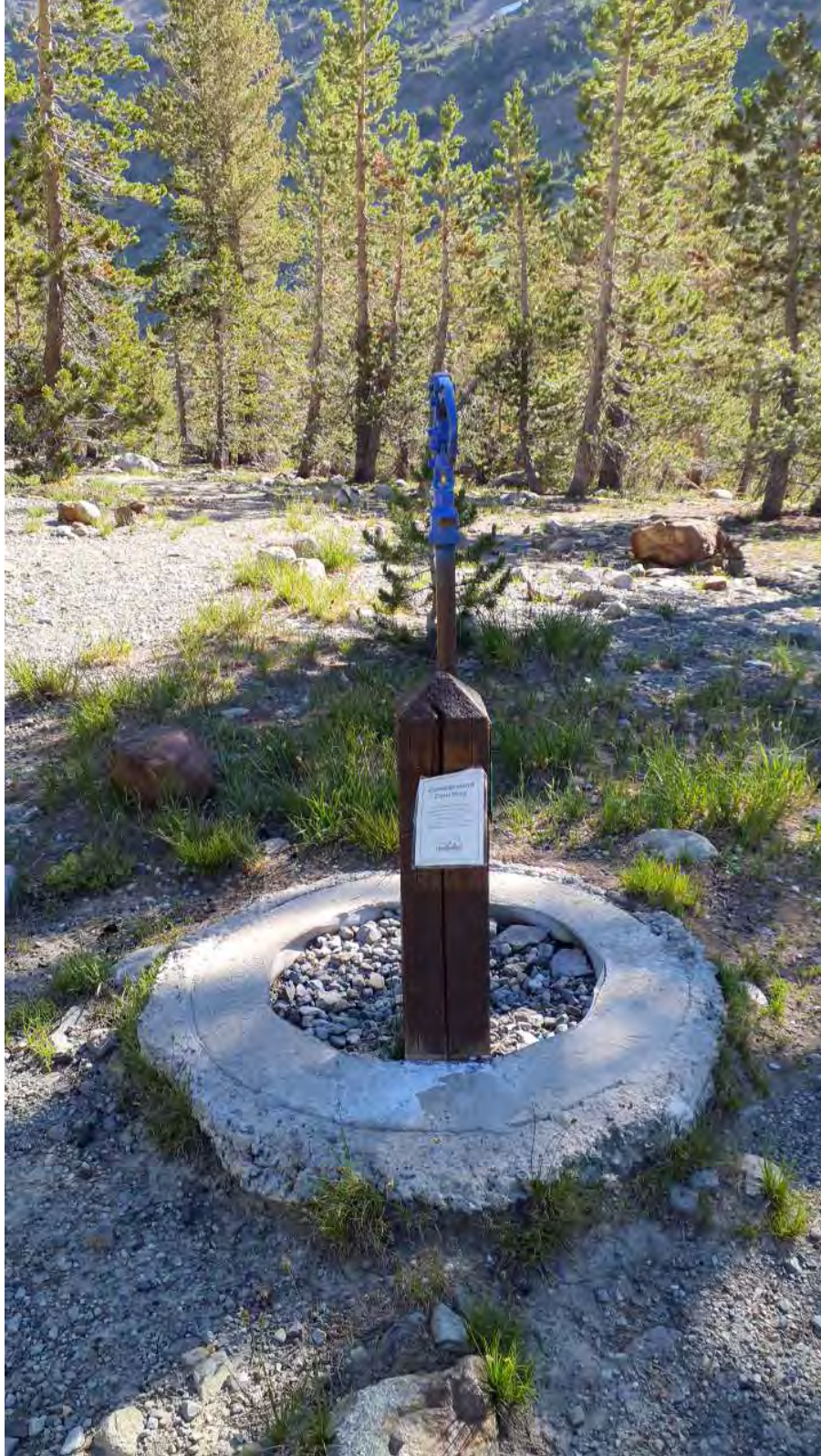
Photo 8. Saddlebag Lake Campground, Potable Water Pump
