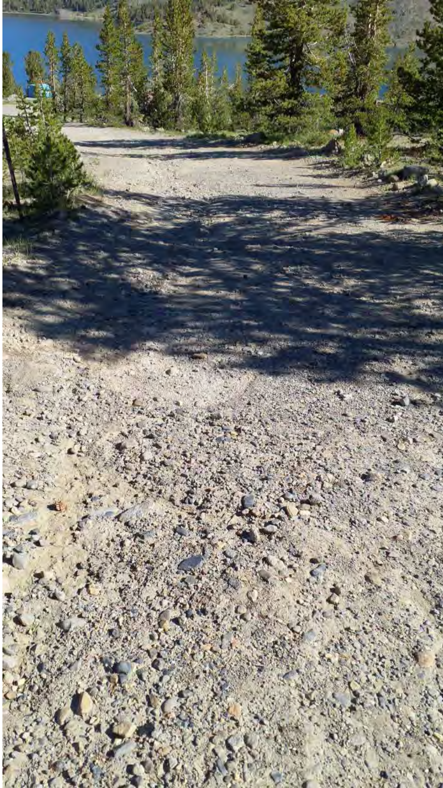
Photo 9. Saddlebag Lake Campground, Erosion
