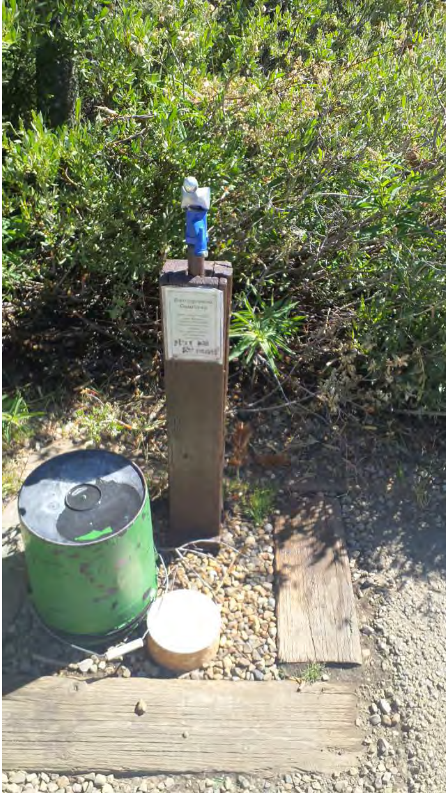
Photo 51. Ellery Lake Campground, Potable Water Pump
