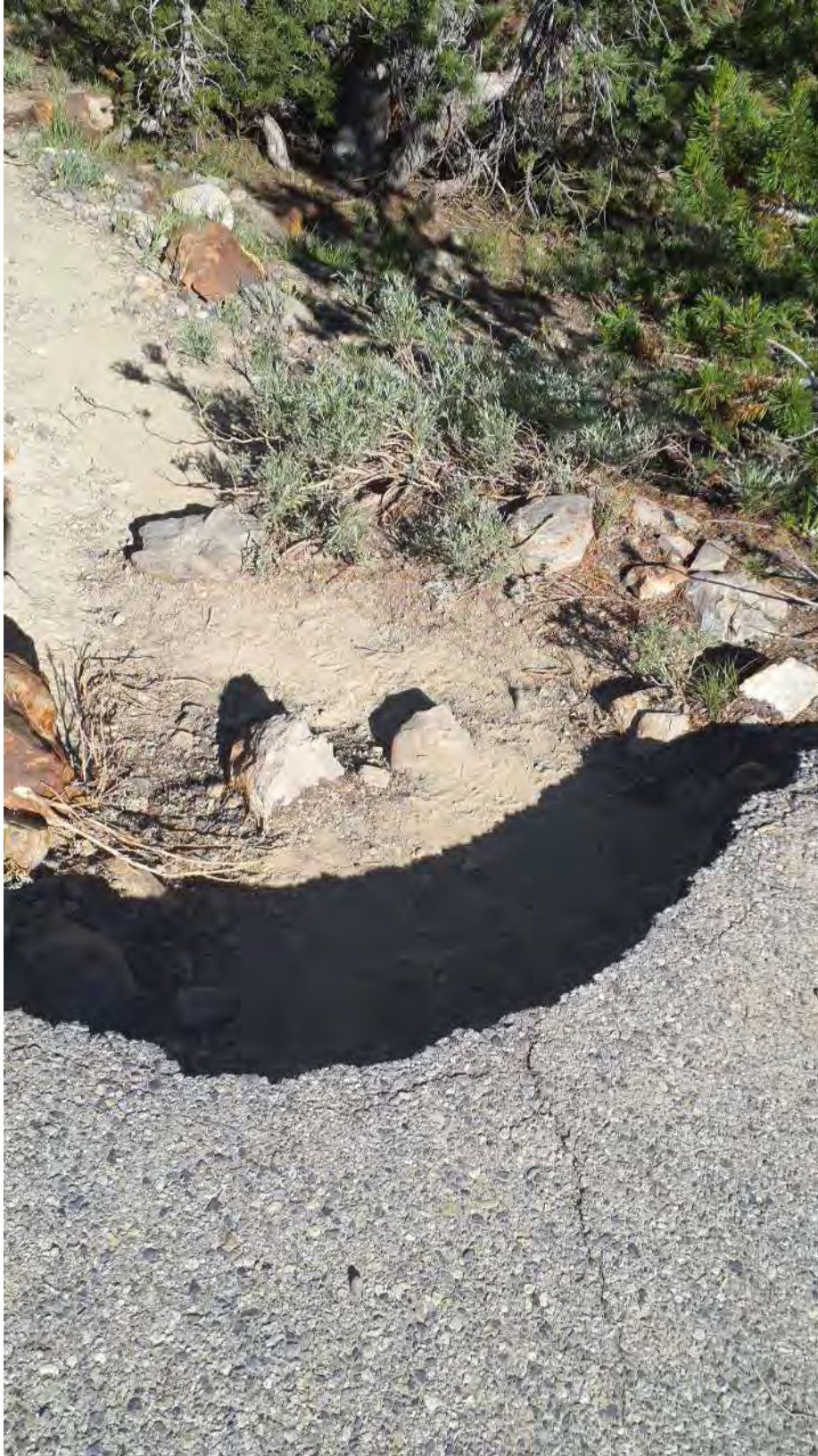
Photo 36. Tioga Lake Campground, Erosion
