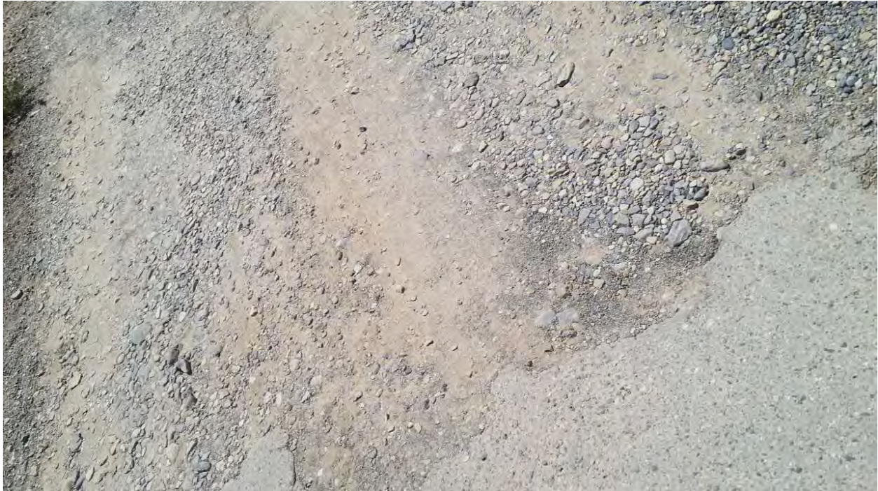
Photo 63. Junction Campground, Erosion
