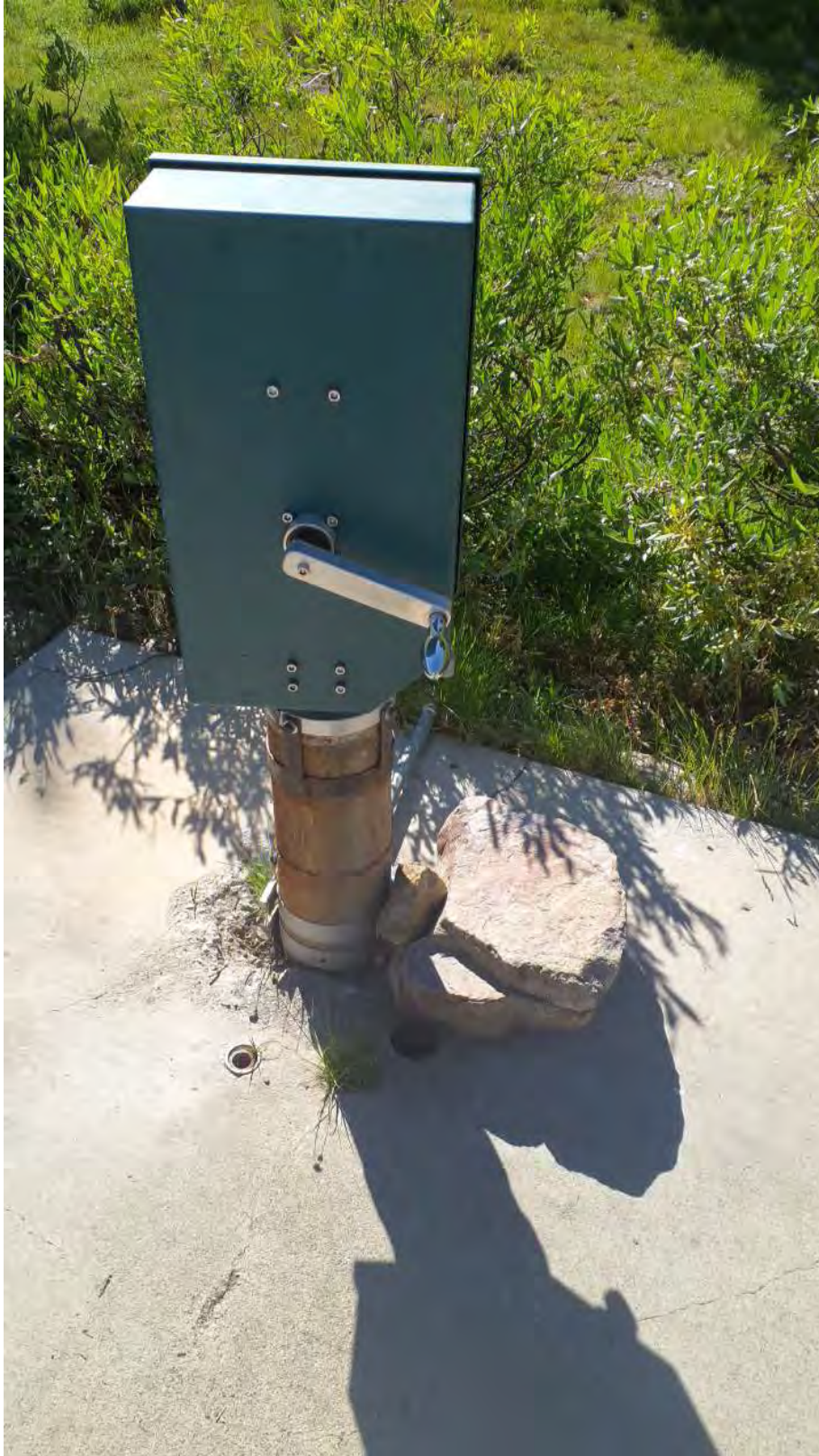
Photo 32. Tioga Lake Campground, Potable Water Pump
