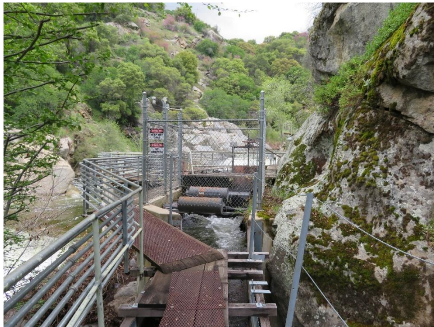
Photo B-8. Kaweah No. 1 Flowline Control Gate Fence with warning signage. Photo taken April 17, 2018.
