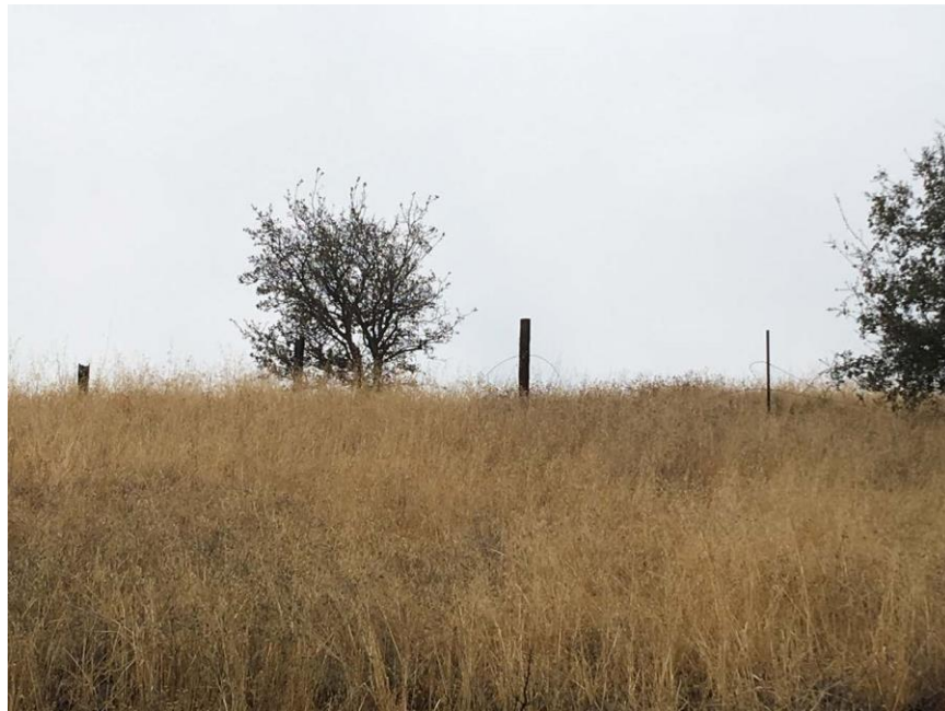
Photo C-4. Poor condition fence along the Kaweah No. 2 Flowline. Photo taken on November 11, 2018.
