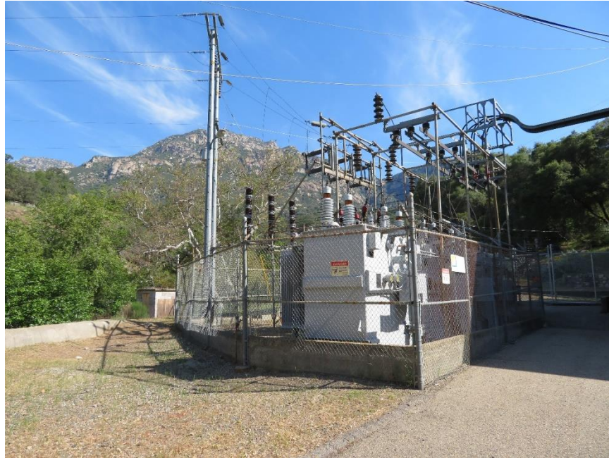
Photo B-19. Kaweah No. 3 Switchyard Perimeter Fence with warning signage. Photo taken April 17, 2018.
