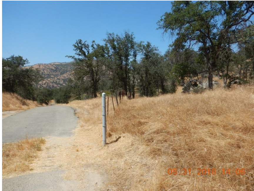
Photo C-3. Poor condition cattle guard (lower left) and fair condition non-Project fence on the Kaweah No. 1 Forebay Road (Photo taken on May 31, 2018).
