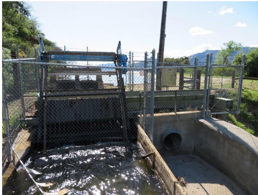
Photo B-18. Kaweah No. 3 Forebay Inlet Trash Rack Fence. Photo taken April 17, 2018.
