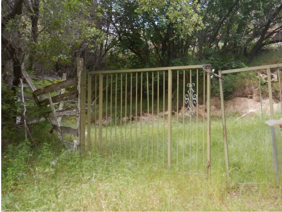
Photo D-13. Kaweah No. 1 Flowline Access Road – Unnamed, road start and gate, poor condition, May 8, 2018
