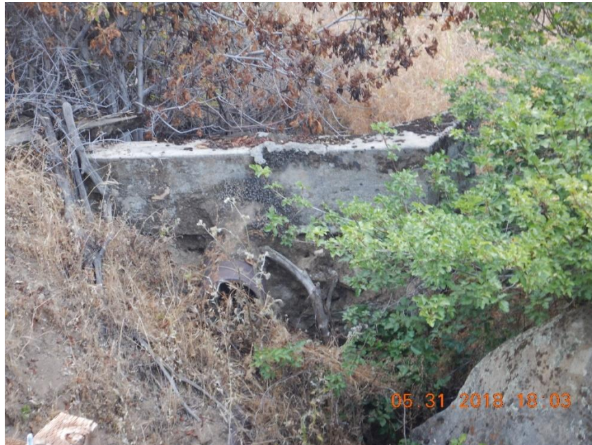
Photo C-6. Concrete structure found along the Kaweah No. 2 Flowline at the location provided by the BLM. Photo taken on May 31, 2018.
