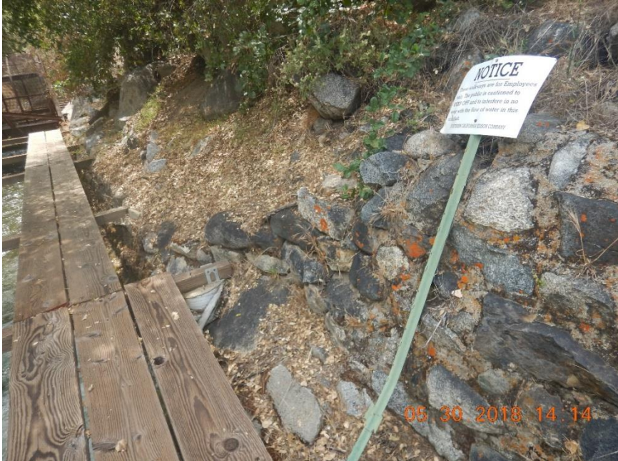
Photo B-5. Kaweah No. 2 Flowline, warning sign, fair condition; wooden planks on walkway, good condition. Photo taken May 30, 2018.
