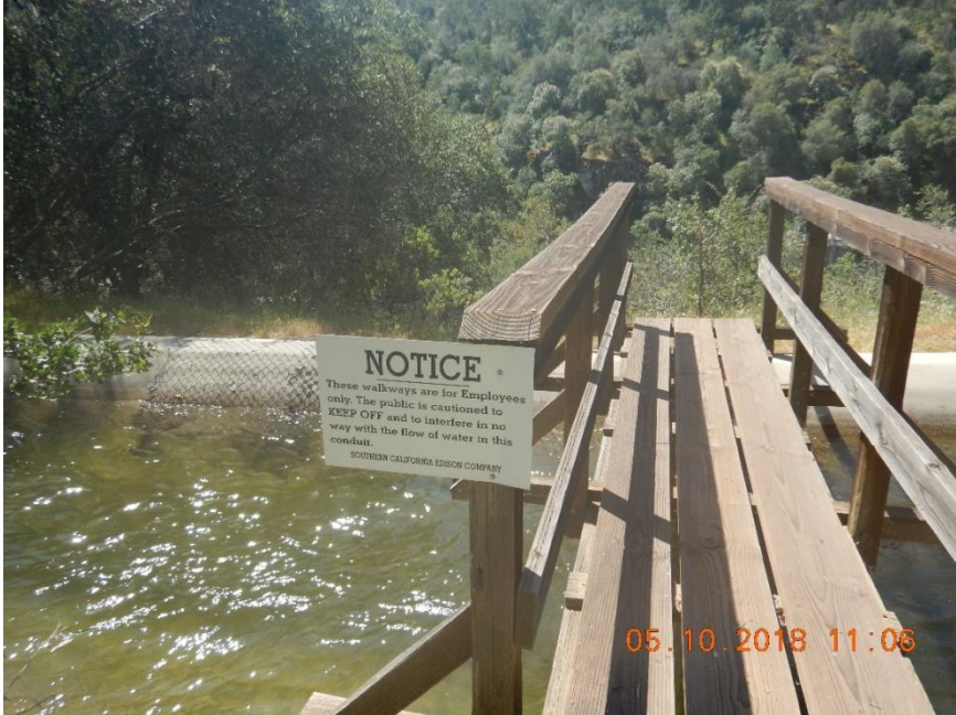
Photo B-1. Kaweah No. 2 Flowline, footbridge with warning sign in foreground and escape fencing in background, all in good condition. Photo taken on May 10, 2018.
