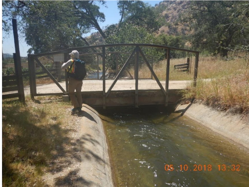
Photo B-17. Kaweah No. 2 Flowline Access Road Bridge Fence (on both sides of bridge crossing). Photo taken May 10, 2018.
