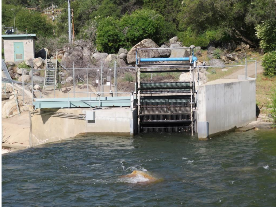
Photo B-5. Kaweah No. 2 Diversion Dam intake structure after 2012 modifications. Photo taken May 8, 2018.
