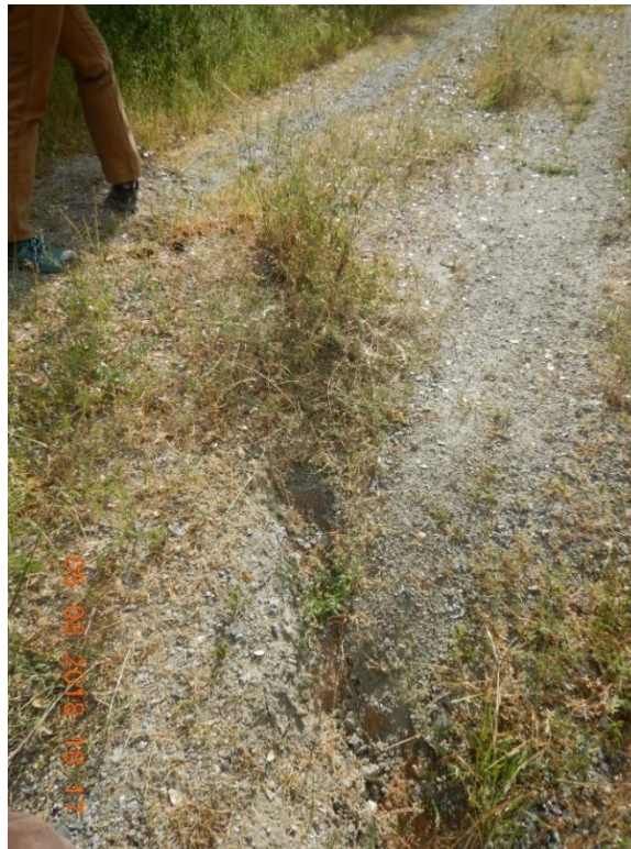
Photo D-14. Kaweah No. 1 Flowline Access Road – Grapevine, example of road damage, May 8, 2018
