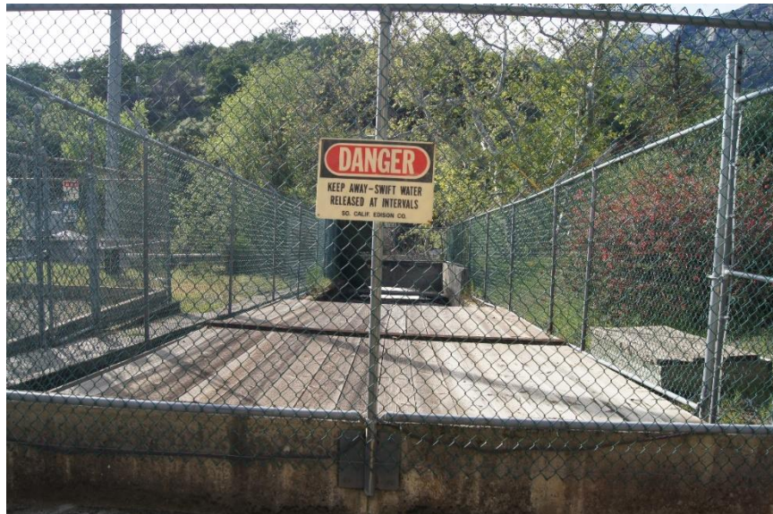
Photo B-20. Kaweah No. 3 Tailrace Channel Fence with warning signage. Photo taken April 17, 2018.
