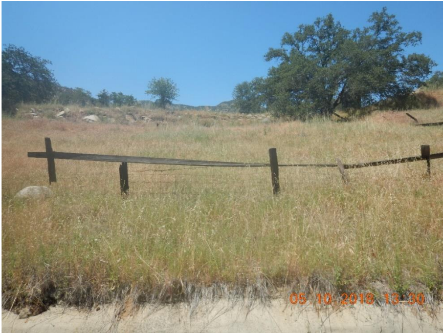
Photo C-2. Non-Project fence along the Kaweah No. 2 Flowline, fence in fair condition. Photo taken on May 10, 2018.
