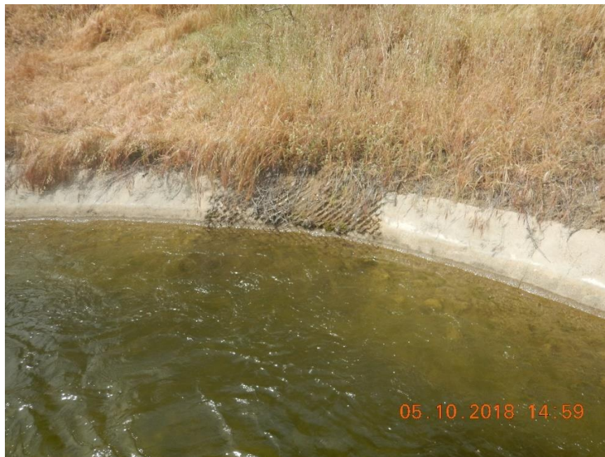
Photo B-4. Kaweah No. 2 Flowline, escape fencing, fair condition. Photo taken May 10, 2018.
