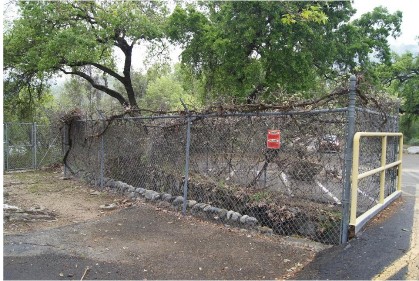
Photo B-15. Kaweah No. 2 Tailrace Channel Fence. Photo taken April 17, 2018.
