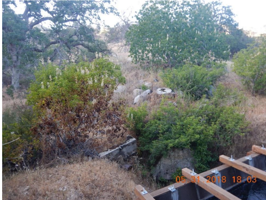
Photo C-7. Concrete structure found along the Kaweah No. 2 Flowline at the location provided by the BLM. Photo taken on May 31, 2018.
