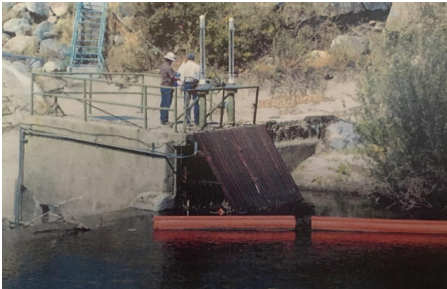
Photo B-4. Kaweah No. 2 Diversion Dam intake structure before 2012 modifications. Date unknown.
