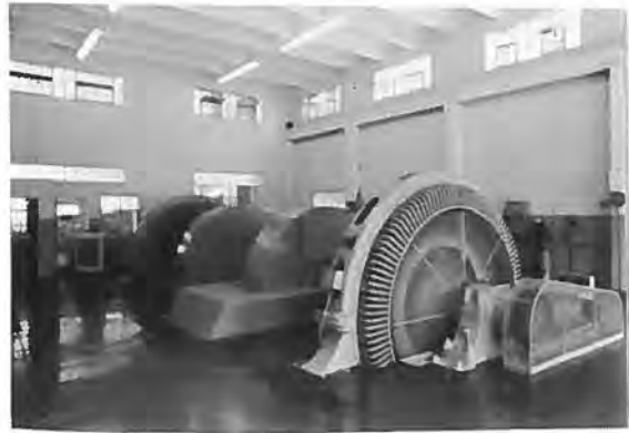
Bldg. 0101, Generator Floor Kaweah Powerhouse No. 3 View to NNW Roll 2, Frame 3, 6-27-89
