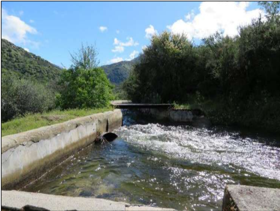
Photograph 9. Marble Fork Siphon emptying into Middle Fork Flowline, camera facing northeast. April 17, 2018.
