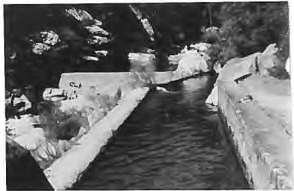
Marble Fork Diversion and Flume Kaweah Powerhouse No. 3 View to NE Roll 2, Frame 20, 6-27-89
