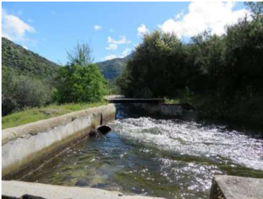
Photograph 5. Junction of Marble Fork Siphon and Middle Fork Flowline, camera facing east, April 17, 2018.
