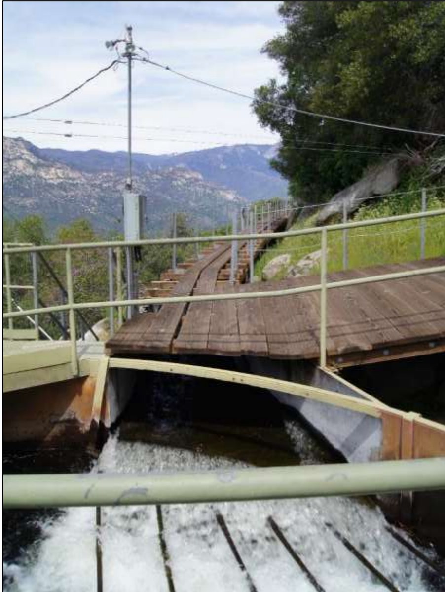
Photograph 2. Connection of Kaweah No. 1 Flowline with Kaweah No. 1 Forebay, camera facing northeast. April 18, 2018.
