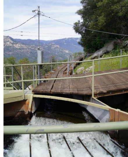
Figure CUL 5-68 Kaweah No. 1 Forebay Tank Communication Line, camera facing east
