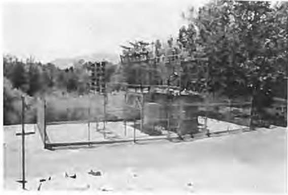
Substation Kaweah Powerhouse No. 2 View to SW Roll 1, Frame 31, 6-27-89
