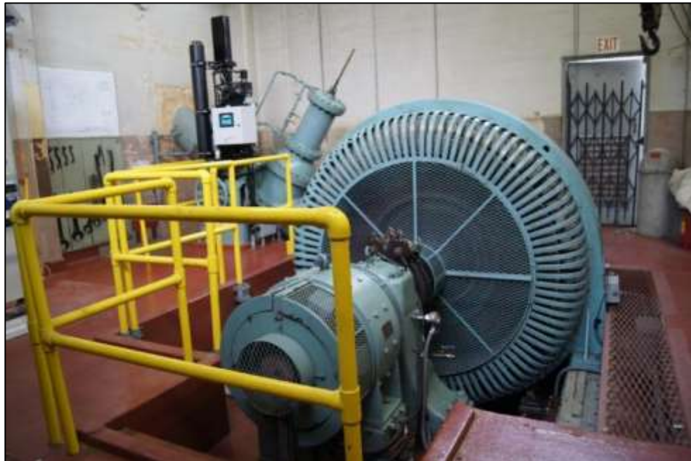
Photograph 5. Interior of powerhouse showing generator, turbine, and penstock, camera facing west, April 18, 2018.
