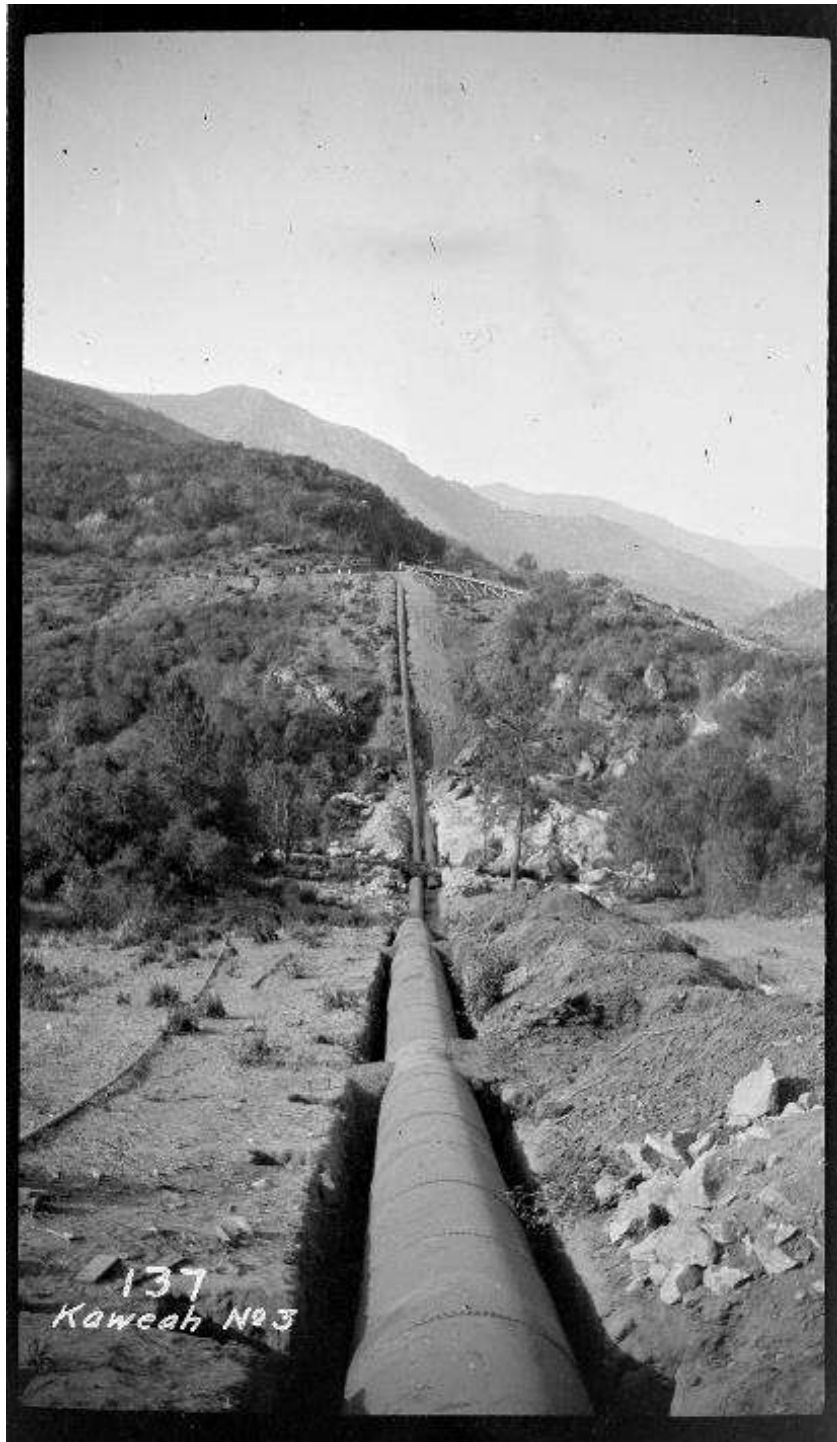
Figure 20: Marble Fork Siphon, circa 1912 (Huntington Digital Library, SCE Photograph Collection, Call Number 04 - 00137)
