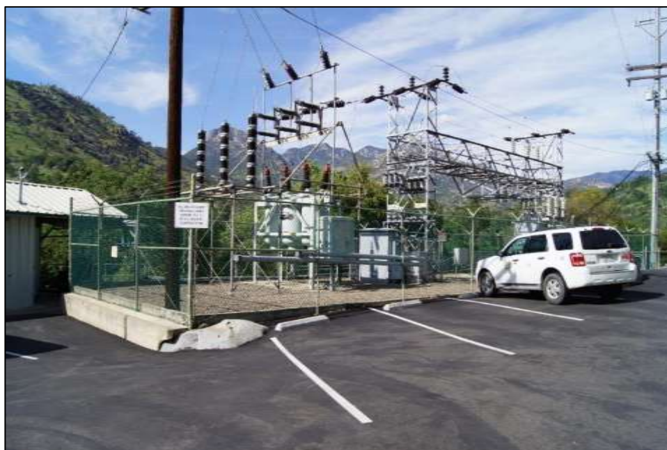
Photograph 7. Kaweah No. 1 Switchyard, camera facing northeast, May 18, 2018.
