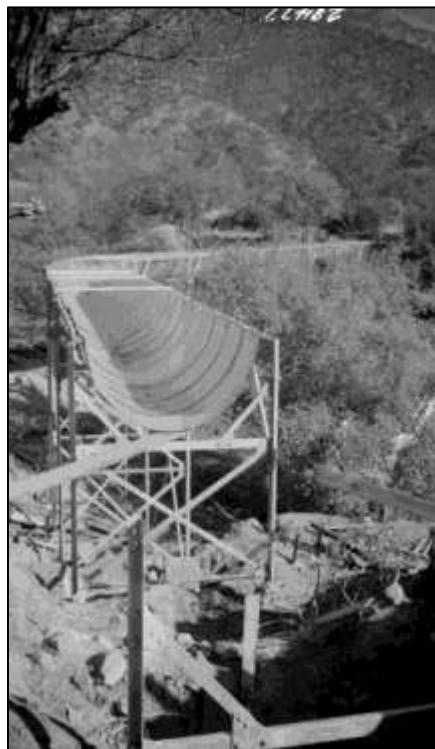
Figure 3. Reconstruction of Kaweah No. 2 Flowline, note metal flume and support structure, 1948 (Huntington Library, Call Number 02 - 28477).
