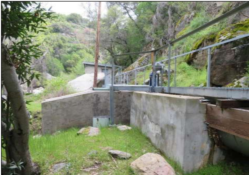
Photograph 9. Modern concrete spillway with gauge house in distance, camera facing southeast. April 18, 2018.
