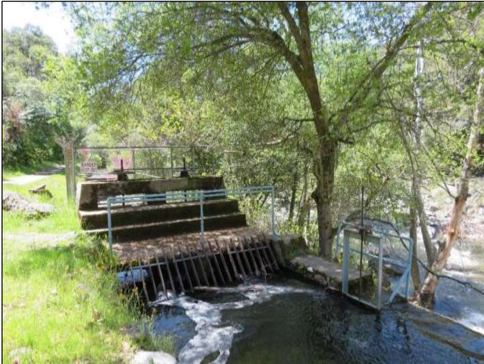
Photograph 6. Trash rack and slide gates at Marble Fork Diversion, camera facing southwest. April 17, 2018.
