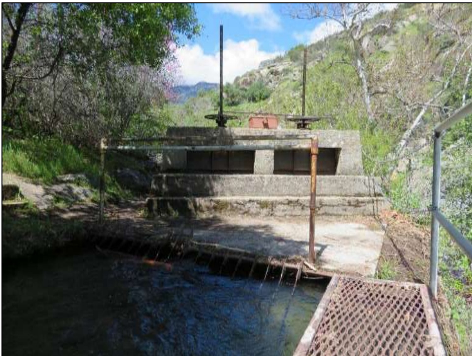
Photograph 5. Middle Fork Diversion trash rack, and slide gates, camera facing west. April 17, 2018.
