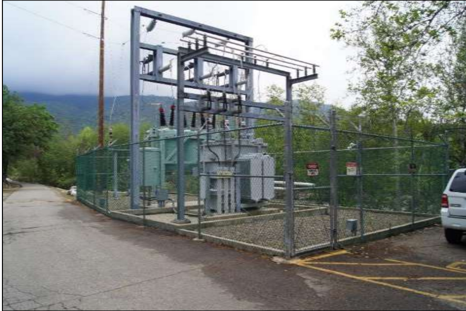
Photograph 8. Kaweah No. 2 Substation, camera facing south. April 19, 2018.
