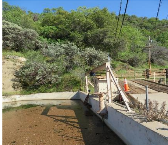
Figure CUL 5-65 Kaweah No. 3 Forebay Outlet, camera facing south
