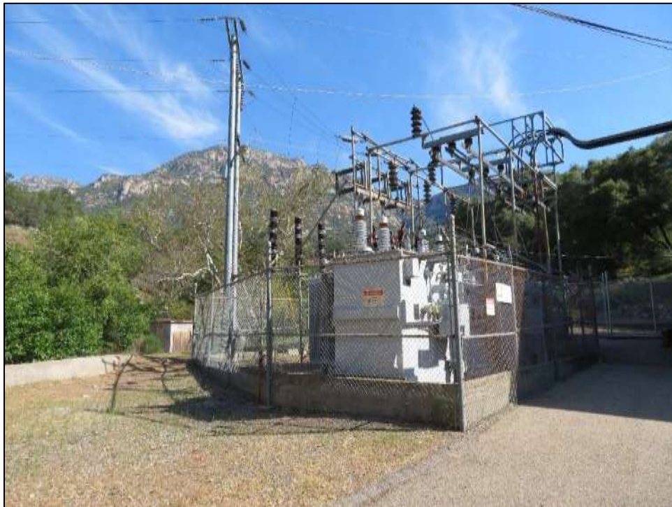
Photograph 8. Kaweah No. 3 Switchyard, note conduit connection, camera facing north. April 18, 2018.
