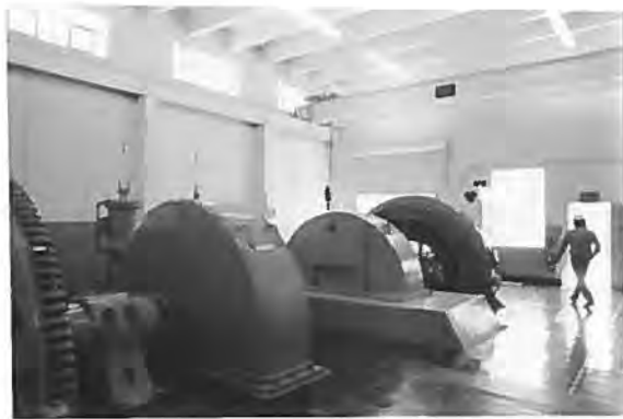
Bldg. 0101, Generator Floor Kaweah Powerhouse No. 3 View to S Roll 2, Frame 5, 6-27-89
