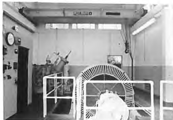
Bldg. 0101, Interior Kaweah Powerhouse No. 1 View to SW Roll 1, Frame 6, 6-27-89
