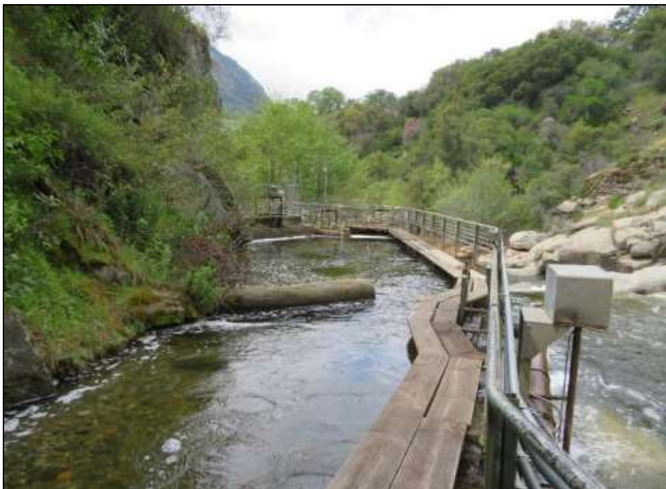
Photograph 5. Kaweah No. 1 Diversion Sandbox showing interior diversion structure, walking platform, and slide gates, camera facing southwest. April 18, 2018.
