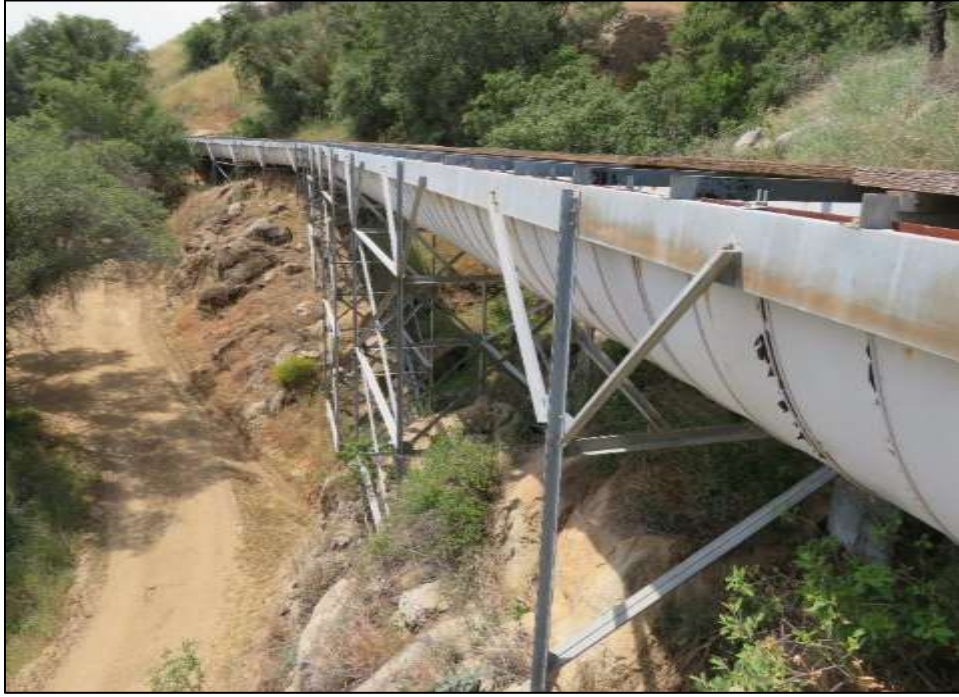
Photograph 4. Flume span along Kaweah No. 2 Flowline, note replacement metal support structure, camera facing northwest. May 8, 2018.
