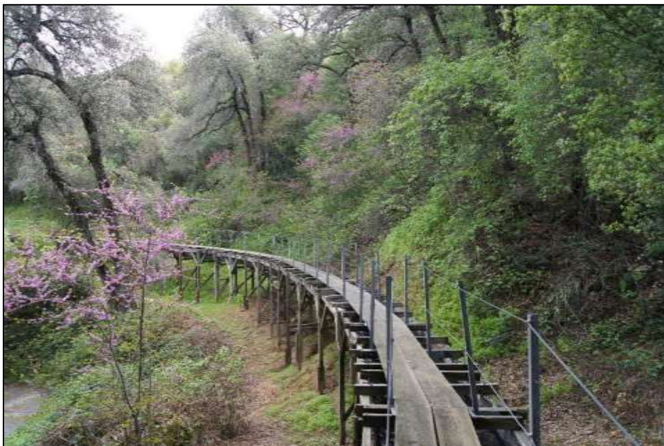
Photograph 3. Kaweah No. 1 Flowline, note post and beam support structure, camera facing northeast. April 18, 2018.
