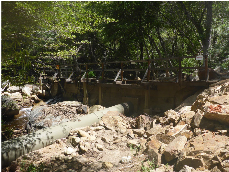
Figure A-18. Downstream side of Salmon Creek Diversion Dam with coarse colluvium from minor rockfall erosion along Left (south) channel margin (view looking upstream).
