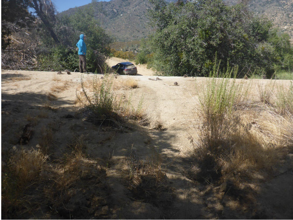
Figure A-11. Tunnel 6/7 Spoil Site showing exposed tunnel section built through drainage swale; upslope side filled to top of tunnel with sediment (view looking downslope from above tunnel).
