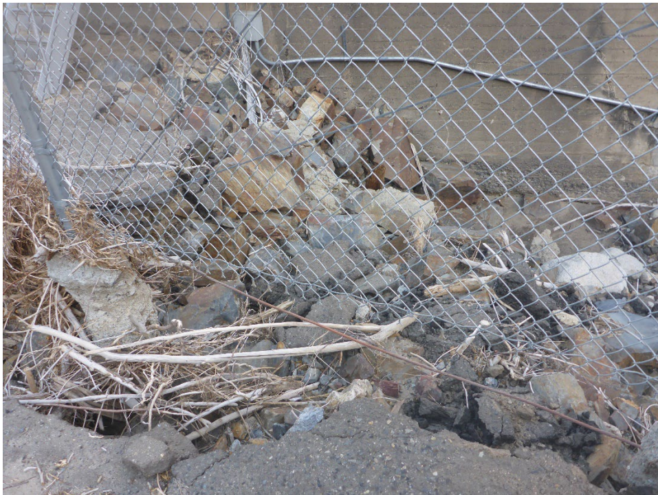
Figure A-4. Erosion and debris near access gate to Fairview Dam Sandbox Facility.
