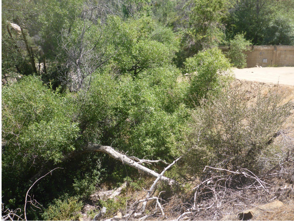
Figure A-20. Left bank (south side) immediately downstream of the exposed flume crossing at Salmon Creek with little-to-no active erosion in historical spoil material.
