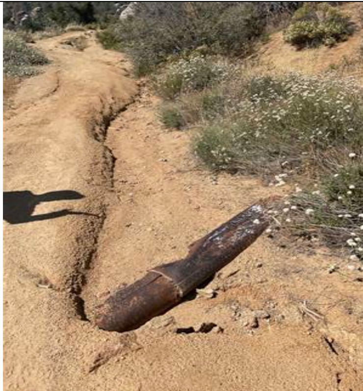
Photograph: 9 Example of unmarked, non-functioning culvert. Rincon Trail Access Road, facing west.
