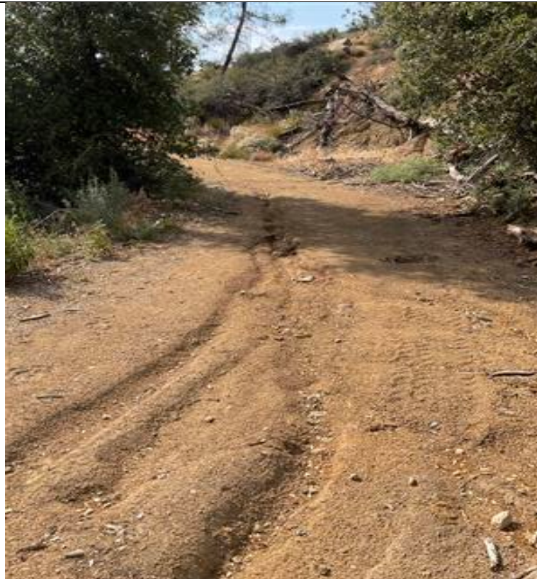
Photograph: 14 Example of erosion rill, the most common erosion feature observed in the field.
