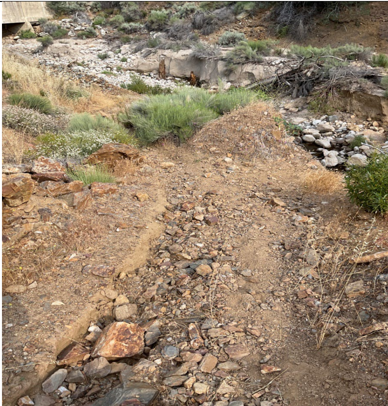
Photograph: 13 Where bridge used to be at Tunnels 10-12 Access Road. Facing southeast.
