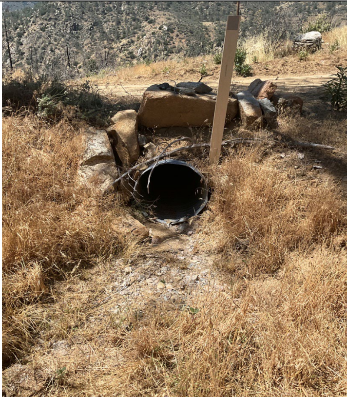
Photograph: 6 Example of culvert categorized as “No Apparent Concern”, inlet side, facing west.
