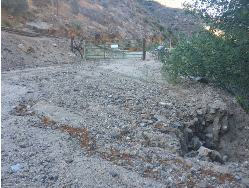
Figure A-5. Minor surface rilling and road fill prism failure cut into access road to Fairview Dam Sandbox Facility (view looking upslope).
