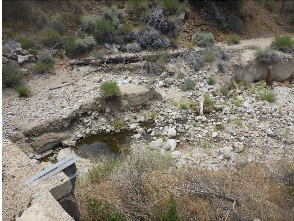
Figure A-25. Close-up view of failed road Crossing at Tunnel 9B/10 Spoil Site (view looking across channel at left bank [south side]).
