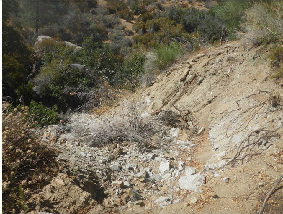
Figure A-13. Small failure in outboard edge of spoil pile fill pad at Tunnel 6/7 Spoil Pile Site; erosional feature located near the farthest downstream edge of spoil pile.
