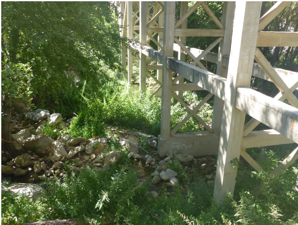
Figure A-44. Concrete footings of elevated flume with minor erosion and sedimentation at Corral Creek crossing.
