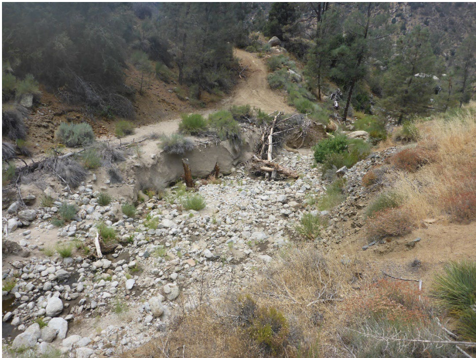
Figure A-24. Failed road crossing at Tunnel 9B/10 Spoil Site (view looking across channel at left bank [south side]).
