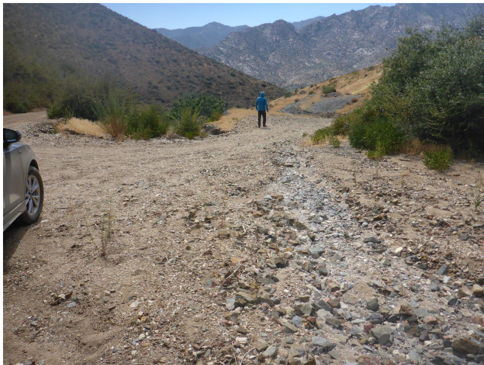
Figure A-50. Tunnel 18/19 Spoil Site with moderate surface erosion of spoil caused by disrupted surface drainage patterns from exposed tunnel section (view from downstream).
