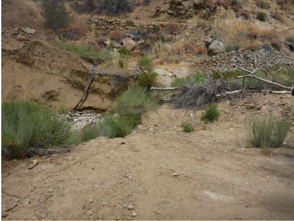
Figure A-23. Failed road crossing at Tunnel 9B/10 Spoil Site (view looking across channel at right bank [north side]).
