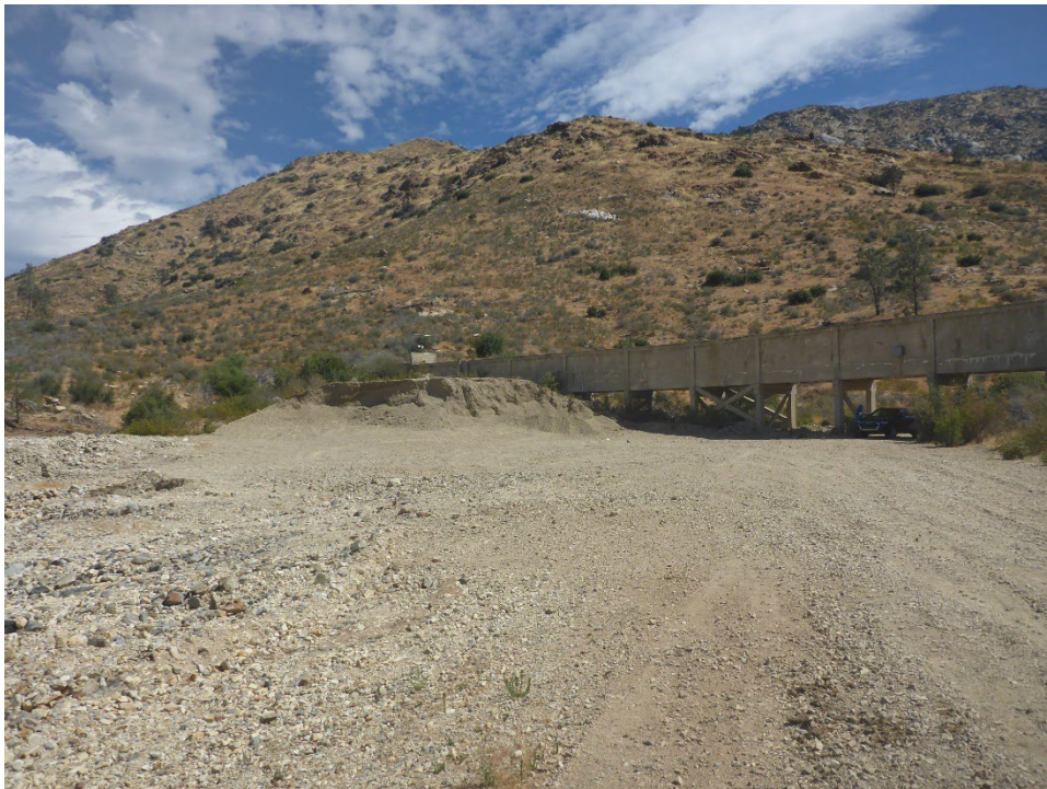
Figure A-42. Spoil material and large pad at Corral North Tunnel 17 Spoil Site. Aggregate stockpile adjacent to exposed tunnel structure in foreground likely imported material for road maintenance.
