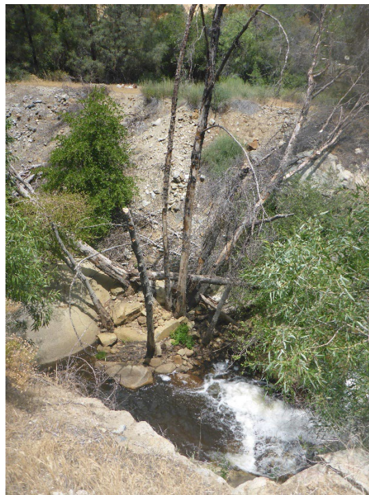
Figure A-20. Right Bank (north side) immediately downstream of the exposed flume crossing at Salmon Creek with little-to-no active erosion in historical spoil material.
