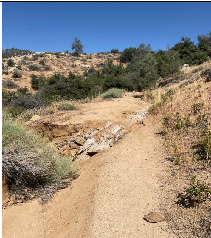
Photograph: 10 Section of Rincon Access Trail Road that is not passable due to erosion concerns. On the east side of Rincon Access Trail road, facing west.
