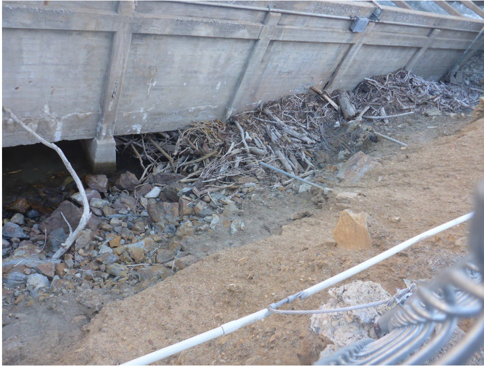
Figure A-3. Close-up view of erosion and debris along inboard edge of Fairview Dam Sandbox Facility near the failed (non-Project) Mountain Highway 99 culvert location.
