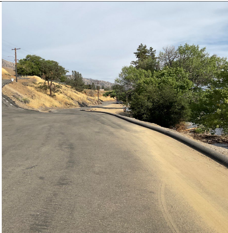
Photograph: 3 Example of Project Access Road in “Good Condition”. Kern River No. 3 Powerhouse Access Road, facing east.
