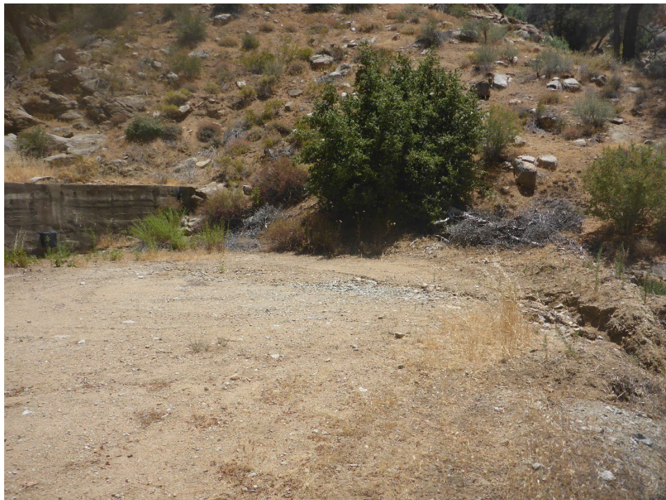
Figure A-30. Tunnel 11 Spoil Site with minor surface erosion along outboard edge of roadbed built on spoil pile pad (view looking upslope).
