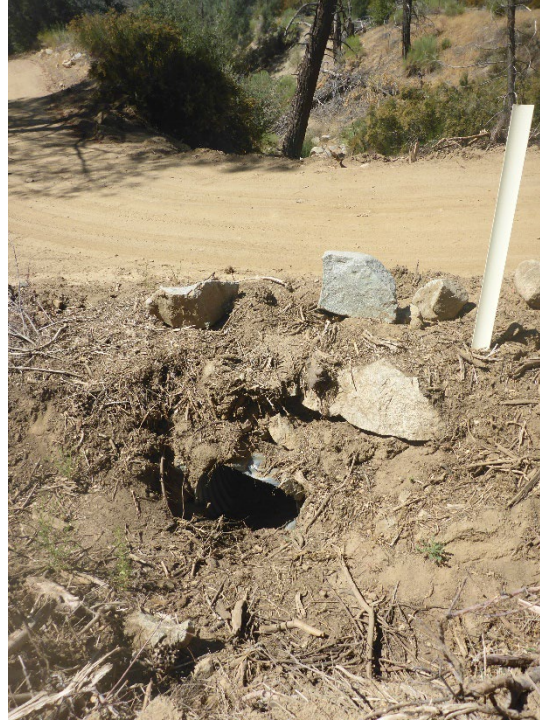
Figure A-15. Recently replaced culvert at Tunnel 8A Site (view looking downstream). Figure A-14 Image photographed from center of road (see witness post for reference).
