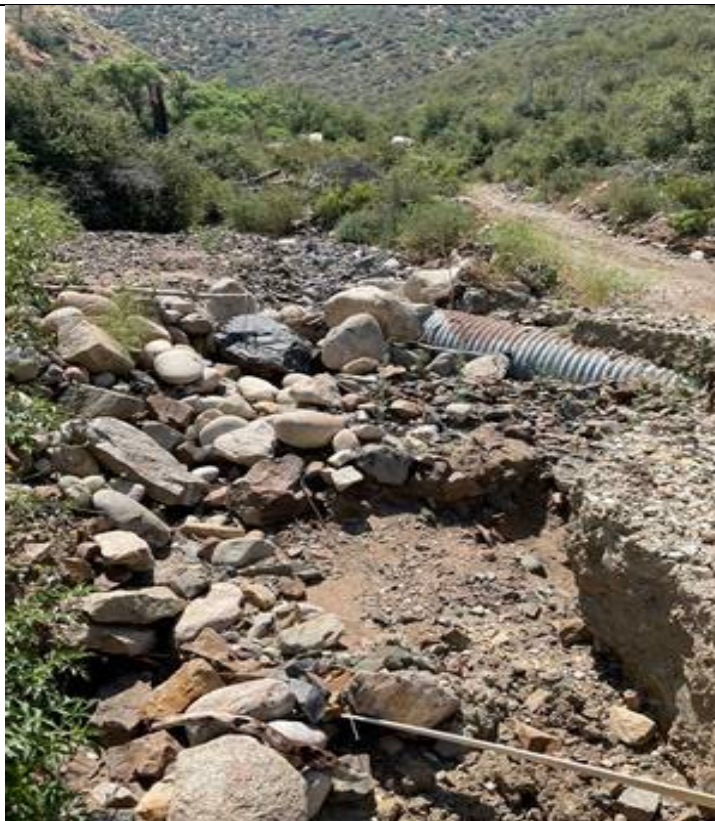
Photograph: 8 Example of culvert categorized as “Concern Likely”, inlet side, facing northeast.
