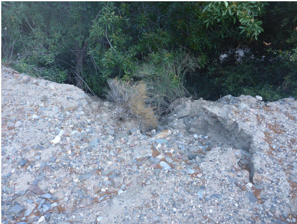
Figure A-6. Minor surface rilling and road fill prism failure cut into access road to Fairview Dam Sandbox Facility (view looking toward river channel, behind vegetation).
