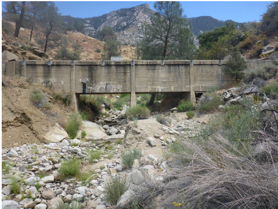
Figure A-22. Failed road crossing at Tunnel 9B/10 Spoil Site (view looking upstream from historical road–stream crossing location).
