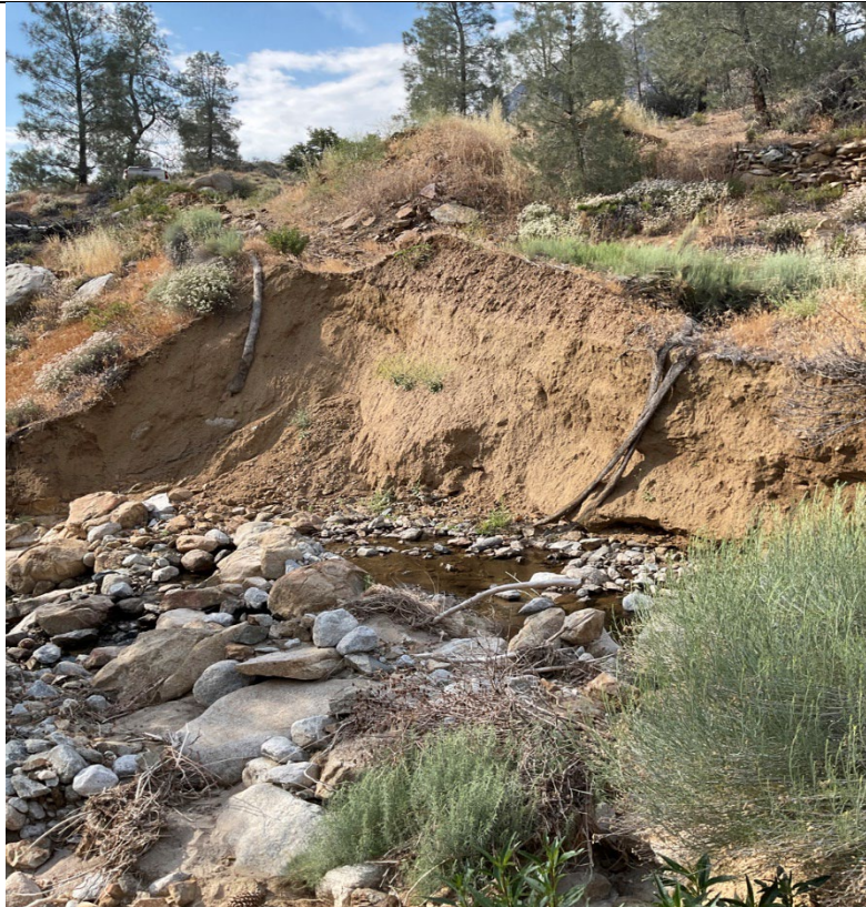
Photograph: 12 Erosion concern, where bridge used to be at Tunnels 10-12 Access Road. Facing northwest.
