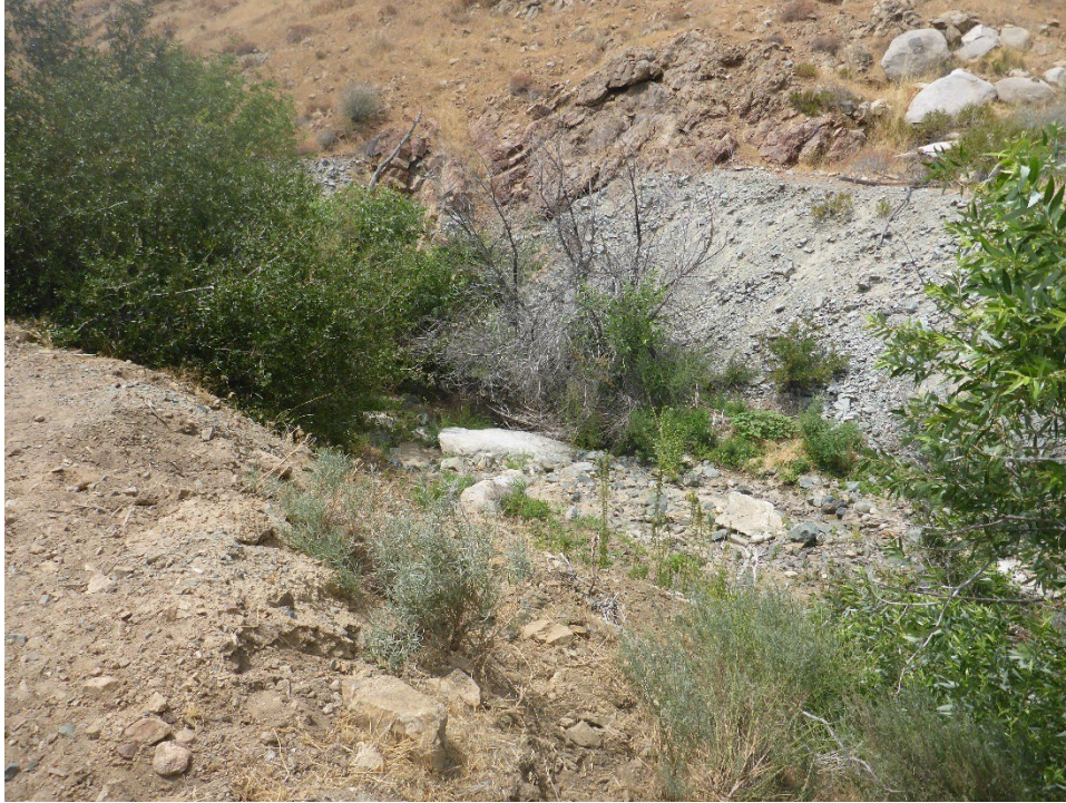
Figure A-35. Spoil Material Exposed along right bank (north side) of Gold Ledge Creek at Tunnel 13/14 Spoil Site; low-to-moderate erosion activity accelerated by cattle crossing trails down embankment (view looking across creek).
