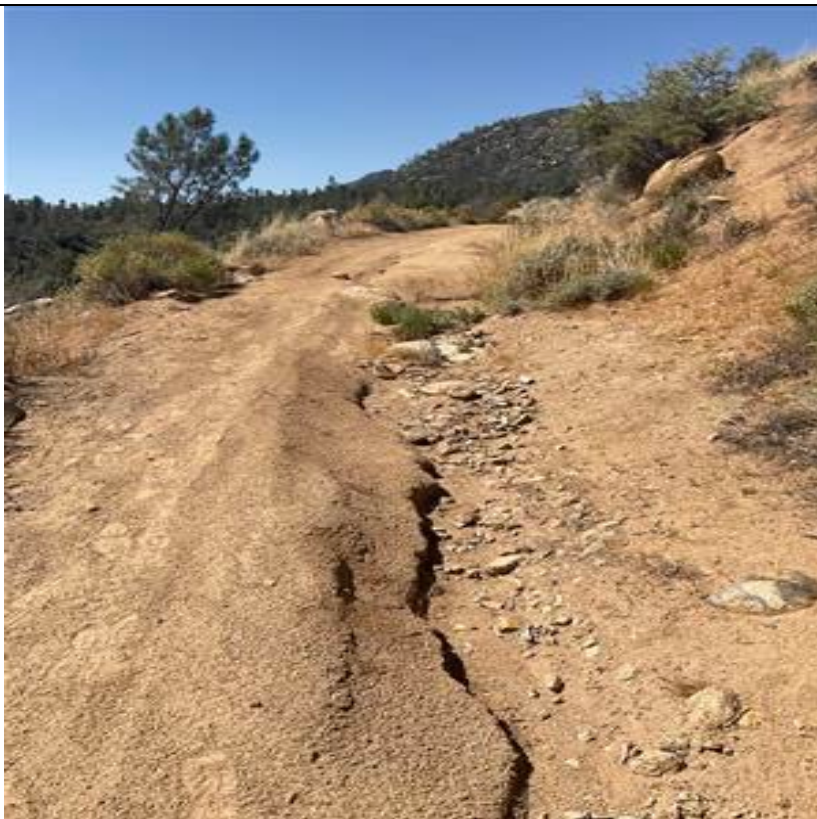
Photograph: 4 Example of road in “poor condition”; erosion gullies, vegetation growing in road, multiple rills. West side of Rincon Trail Access Road, facing west.
