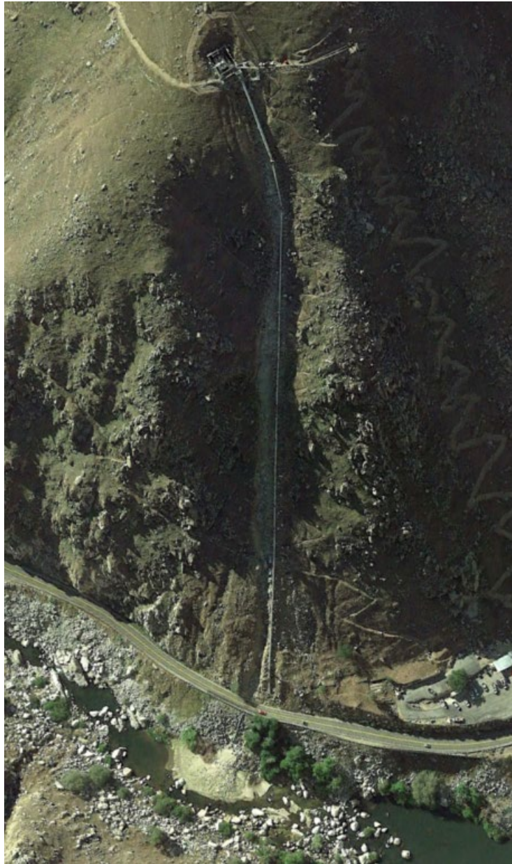
Photo A-22. KR1 Penstock Erosion and Sediment Deposition in the Kern River Channel After the August 20, 2013, Forebay Spill Event (Google Earth Image, Date: 4/15/2014)
