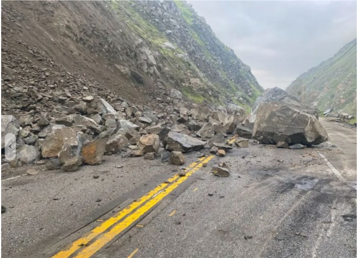
Photo A-24. Debris Slide Closing SR-178 on March 15, 2023 (Caltrans 2023)
