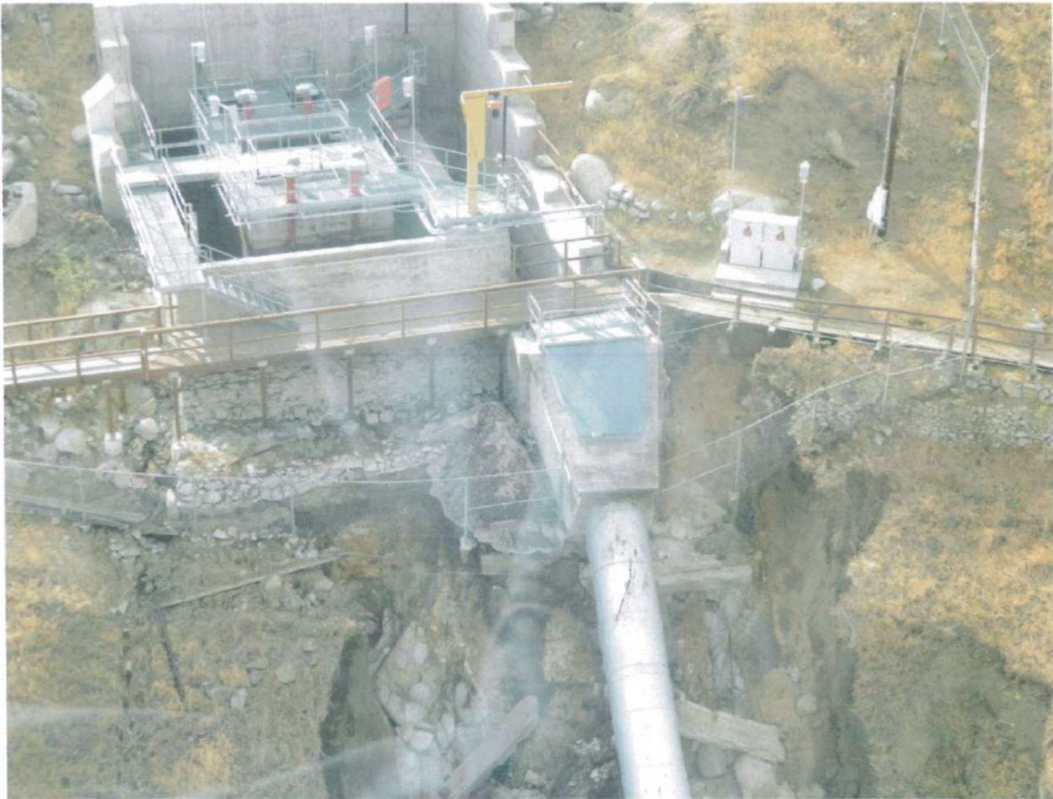
Kern River No. 1 Forebay
