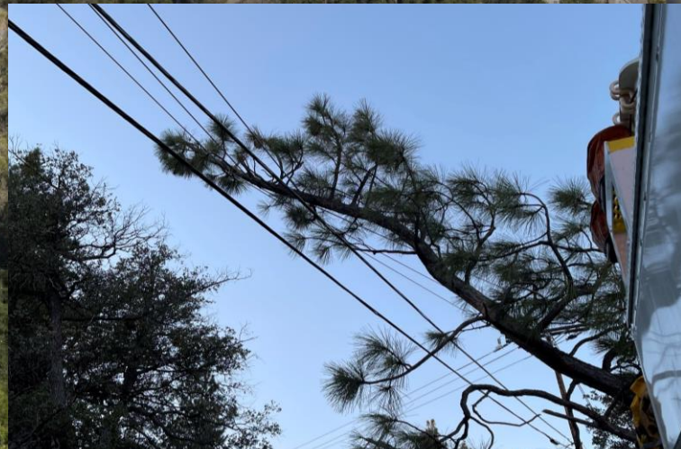
Damage/hazards found after strong winds during PSPS
