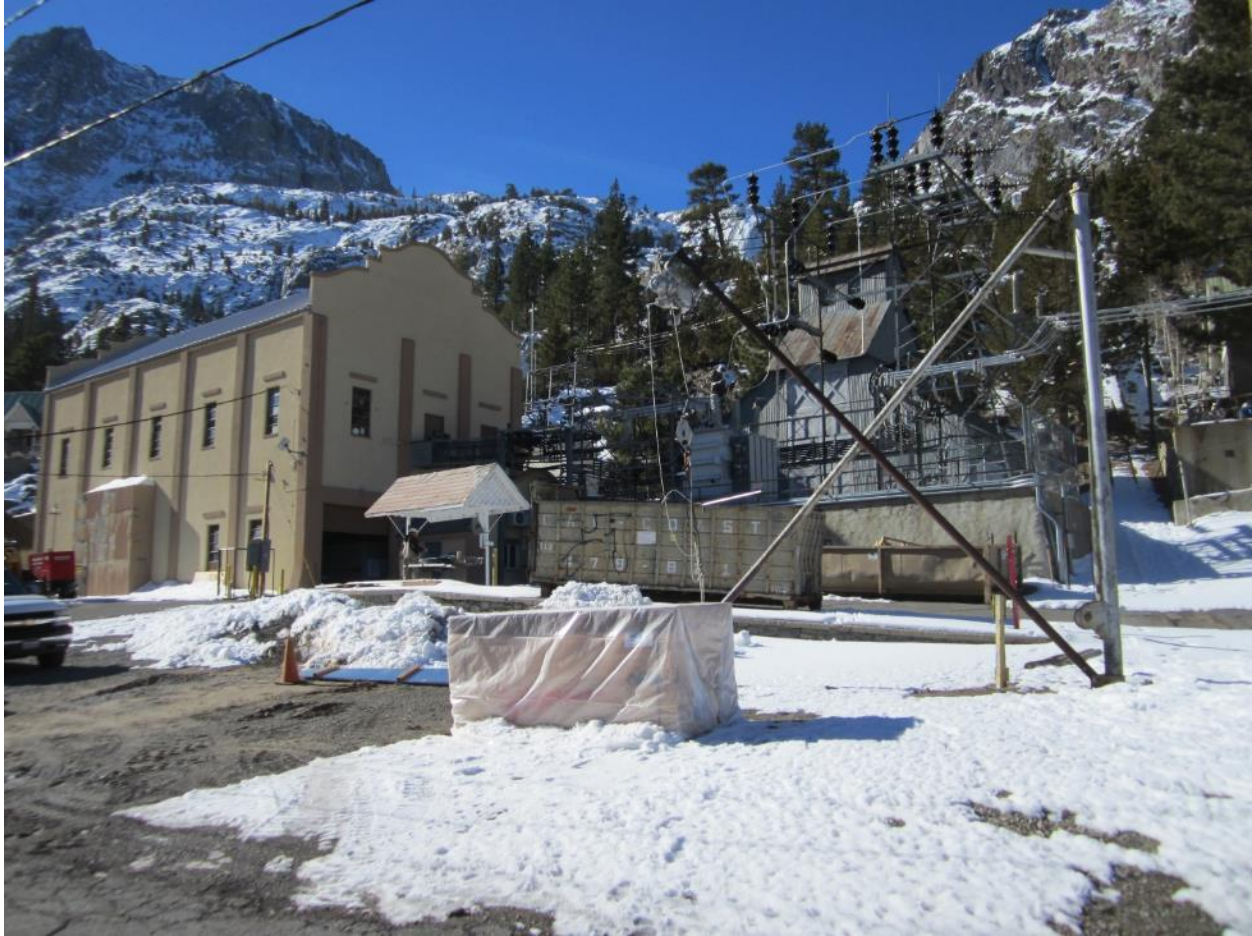
Photo A-9. Rush Creek Powerhouse and Switchyard (non-project facility) (looking west)
