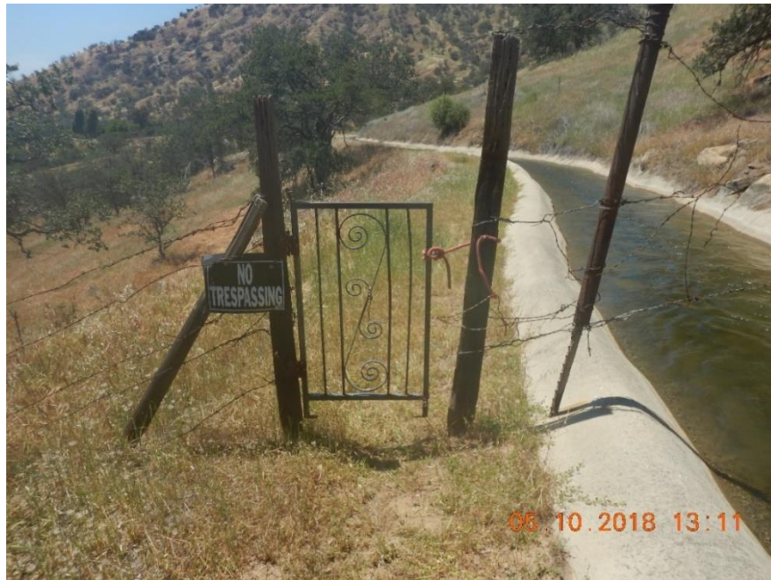
Photo B-6. Kaweah No. 2 Flowline, gate, fair condition; and sign, good condition (May 10, 2018). [#1507]
