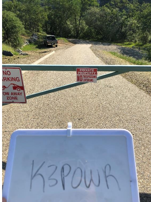
Photo D-1. Kaweah No. 3 Powerhouse Road, road start and gate, good condition, April 24, 2018
