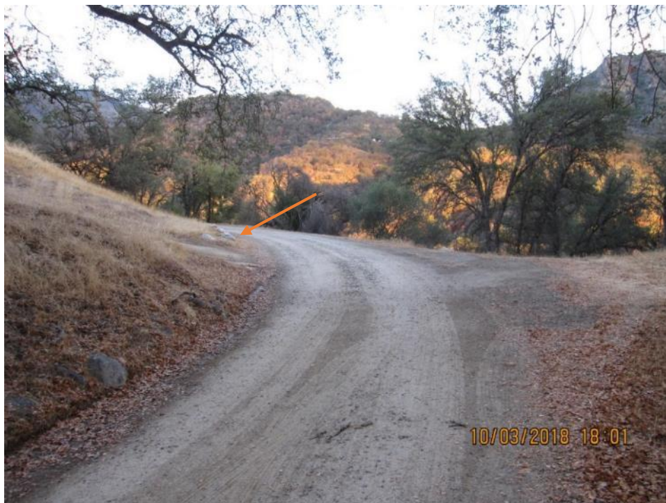
Photo D-16. Intersection of Kaweah No. 2 Flowline East Access Road and Kaweah No. 2 Flowline Access Road – Canal 6 West, example of blind spot, October 3, 2018
