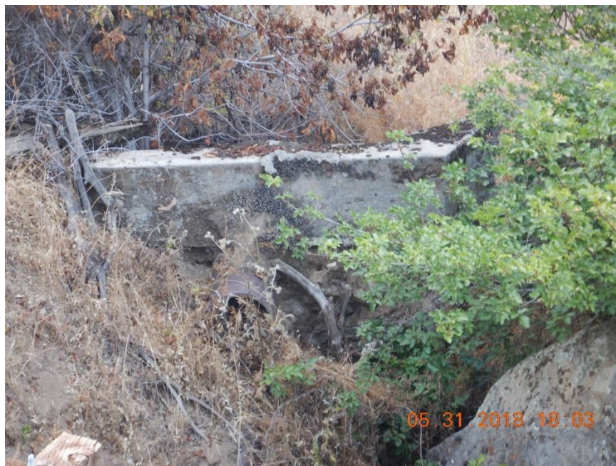
Photo B-16. Kaweah No. 2 Flowline, trough location verification, old feature discovered in trough location (BLM data), poor condition (May 31, 2018). [#1587]
