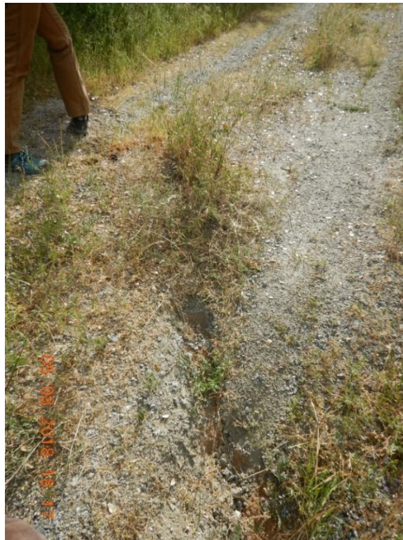
Photo D-14. Kaweah No. 1 Flowline Access Road – Grapevine, example of road damage, May 8, 2018
