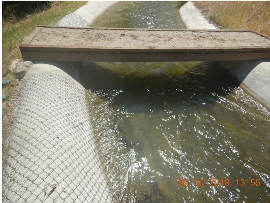
Photo B-3. Kaweah No. 2 Flowline, wildlife bridge and escape fencing, good condition (May 10, 2018). [#1514]
