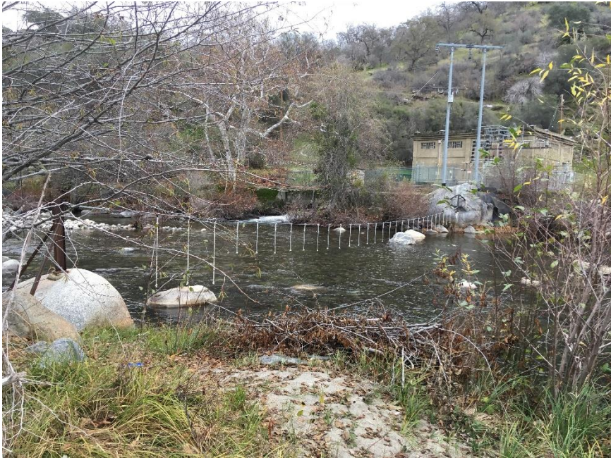
Photo B-9. Kaweah No. 2 Flowline, last chance safety line, good condition, (January 7, 2019). [#10819]
