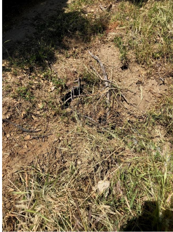
Photo D-7. Kaweah No. 2 Flowline West Access Road, culvert, poor condition, April 24, 2018
