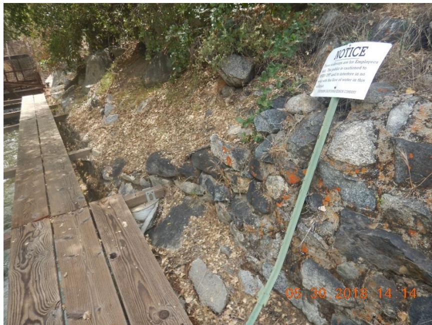
Photo B-8. Kaweah No. 2 Flowline, warning sign, fair condition; wooden planks on walkway, good condition (May 30, 2018). [#1541]
