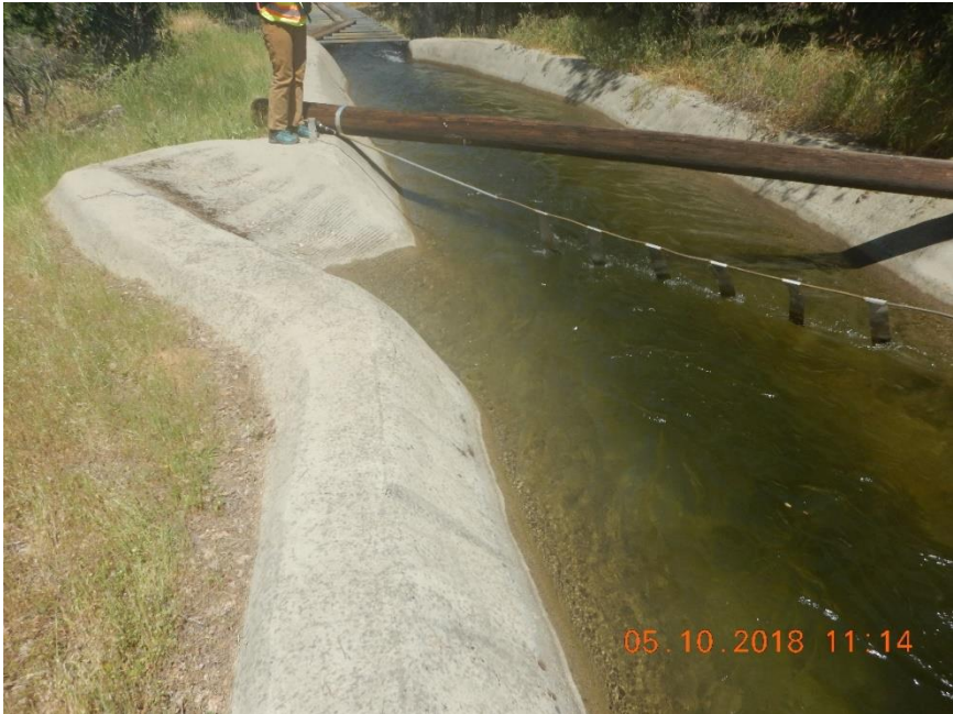
Photo B-2. Kaweah No. 2 Flowline, escape ramp, hazer, and flasher, all in good condition (May 10, 2018). [#1478]
