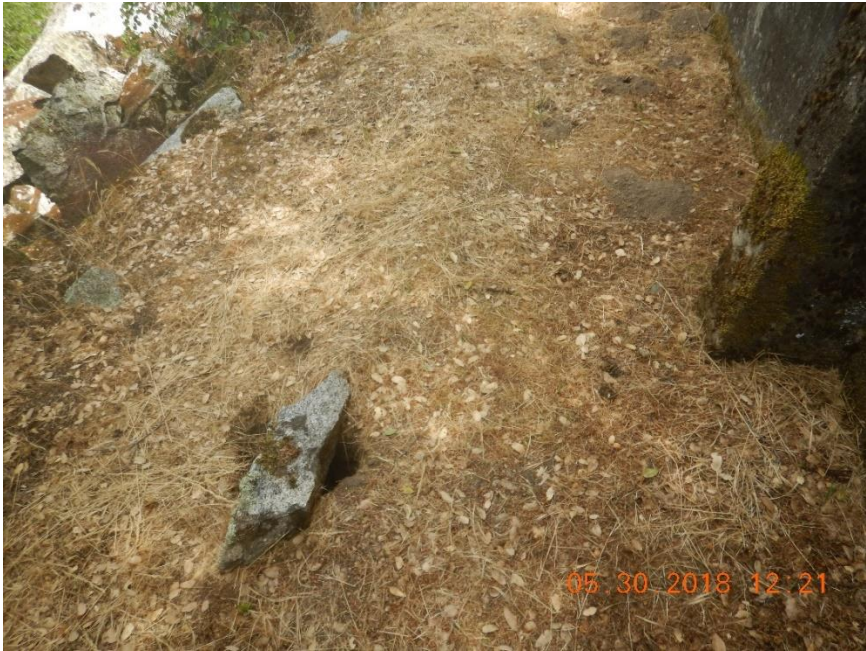
Photo B-10. Kaweah No. 3 Flowline, damage along walkway access of flowline, poor condition (May 30, 2018). [#K3FAT9]
