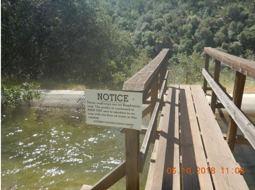
Photo B-1. Kaweah No. 2 Flowline, footbridge with warning sign and escape fencing, both in good condition (May 10, 2018). [#1474]
