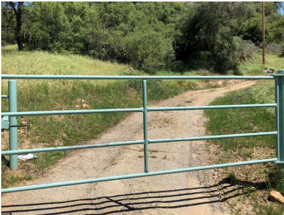
Photo D-12. Kaweah No. 2 Flowline West Access Road, gate, good condition, April 24, 2018
