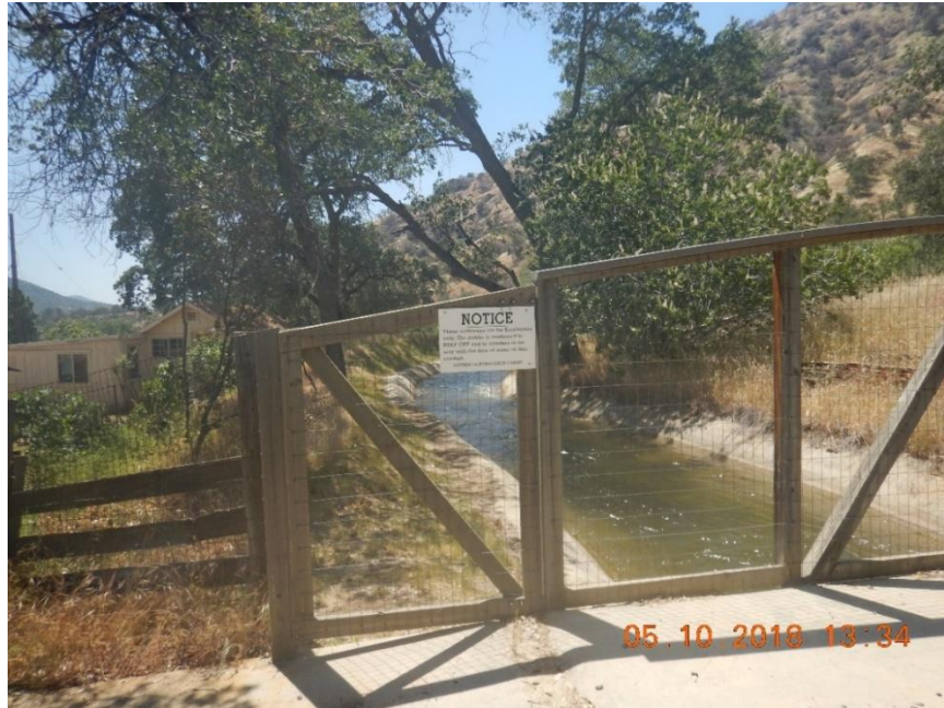
Photo B-11. Kaweah No. 2 Flowline, fence, gate, and signage all in good condition (May 10, 2018). [#1511]
