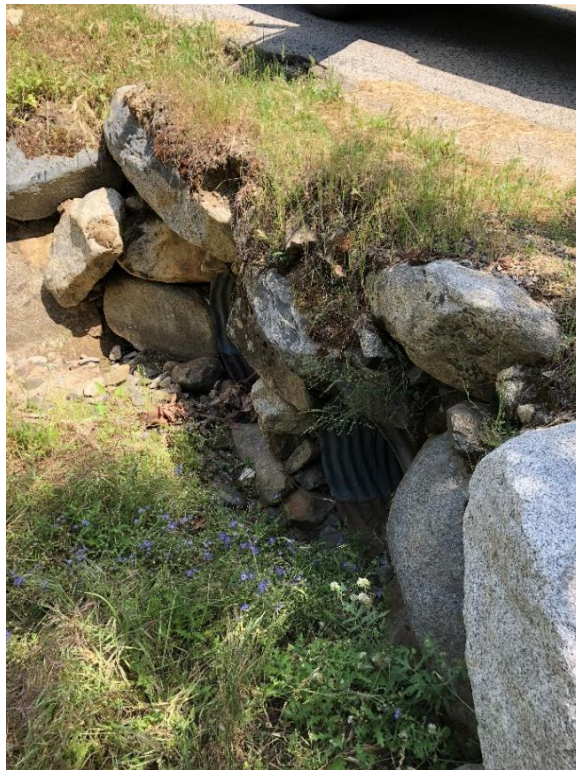
Photo D-6. Kaweah No. 2 Flowline East Access Road, culvert, good condition, April 25, 2018
