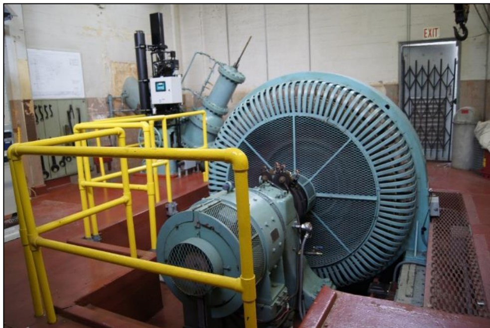
Photograph 5. Interior of powerhouse showing generator, turbine, and penstock, camera facing west, April 18, 2018.
