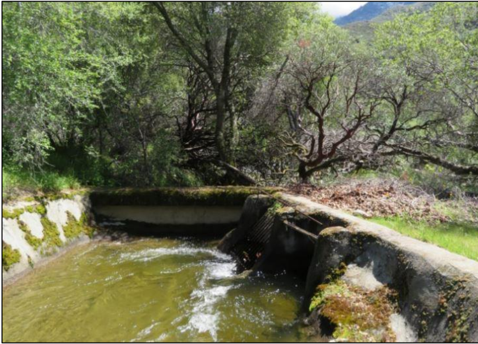
Photograph 6. End of Marble Fork Conduit and headgate for Marble Fork Siphon, camera facing east. April 17, 2018.
