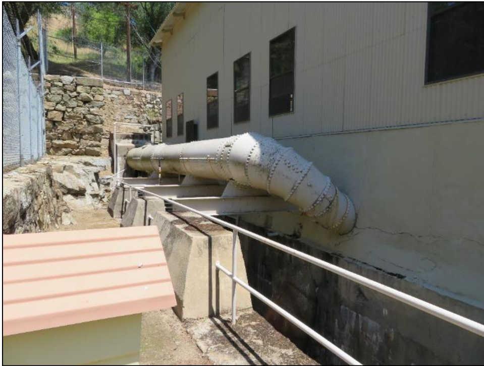
Photograph 6. North side of Kaweah Powerhouse No. 2 showing penstock, camera facing northeast. April 19, 2018.
