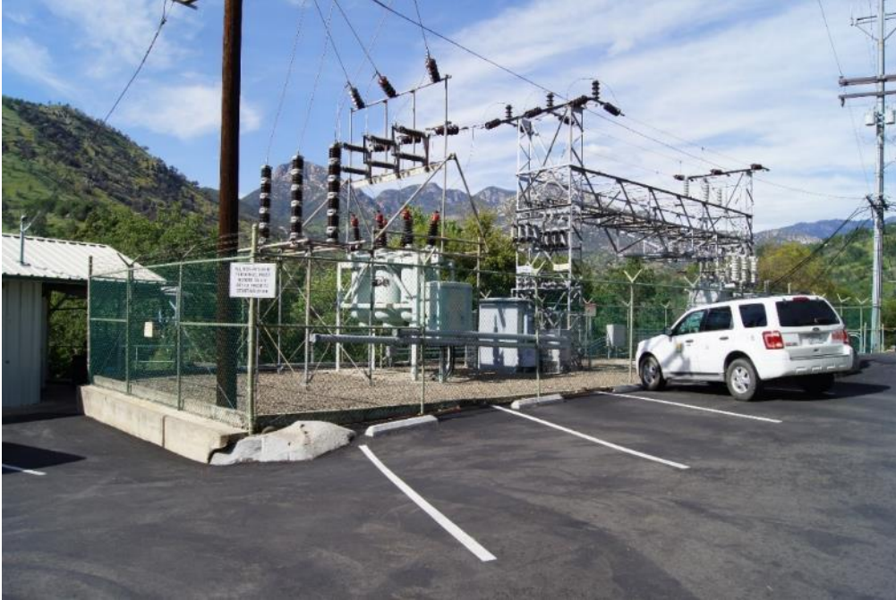
Figure CUL 5-31 Kaweah No. 1 Switchyard, camera facing northeast
