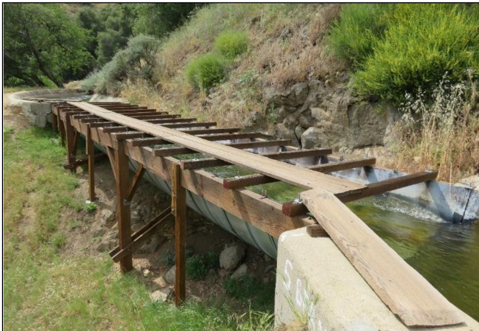
Photograph 5. Flume span along Kaweah No. 2 Flowline showing wood support structure, camera facing northwest. May 8, 2018.
