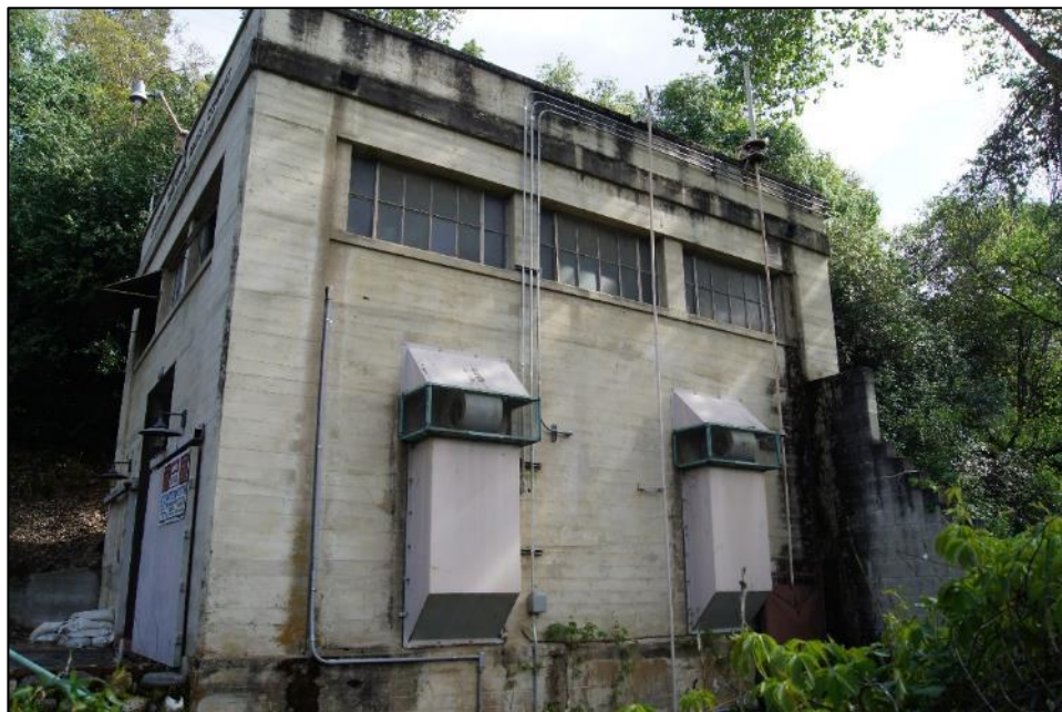
Photograph 9. North side of powerhouse showing air ducts, camera facing south, April 18, 2018.
