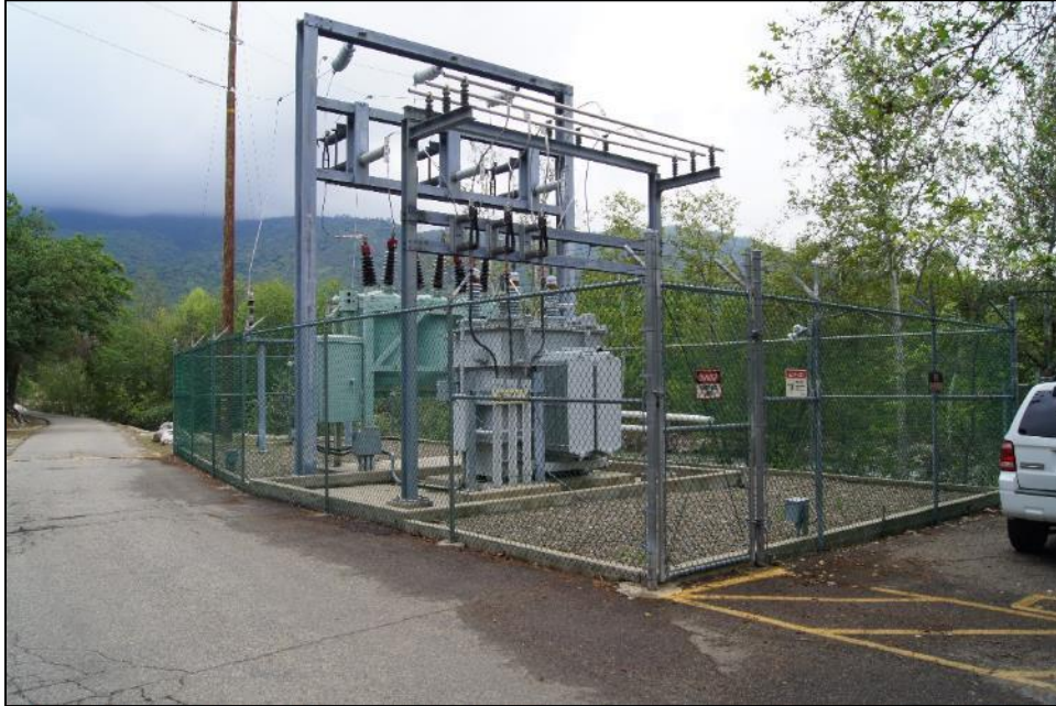
Photograph 8. Kaweah No. 2 Substation, camera facing south. April 19, 2018.
