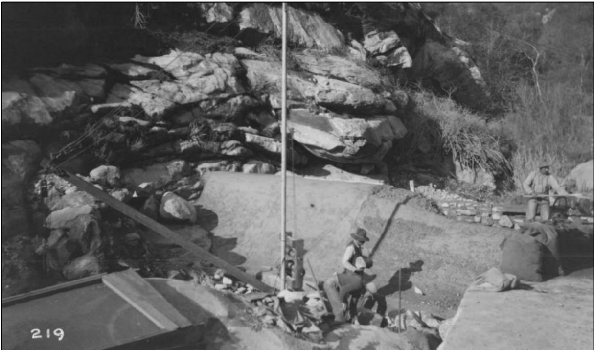
Figure 1. Construction crew at Marble Fork Diversion Dam, ca. 1912 (Huntington Library, Call Number 04 - 00219).
