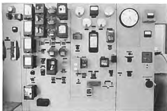
Bldg. 0101, Control Panel Kaweah Powerhouse No. 1 View to SE Roll 1, Frame 4, 6-27-89
