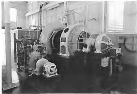
Bldg. 0101, Generator Floor Kaweah Powerhouse No. 2 View to W Roll 1, Frame 26, 6-27-89
