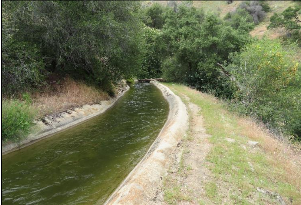
Photograph 2. Concrete lined ditch segment of Kaweah No. 2 Flowline, camera facing northeast. May 8, 2018.
