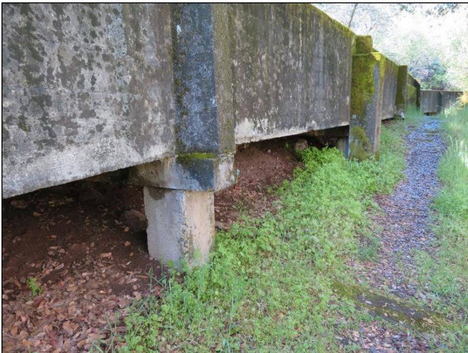
Photograph 5. Footing on Middle Fork Flowline flume, note replacement footing, camera facing west. April 17, 2018.
