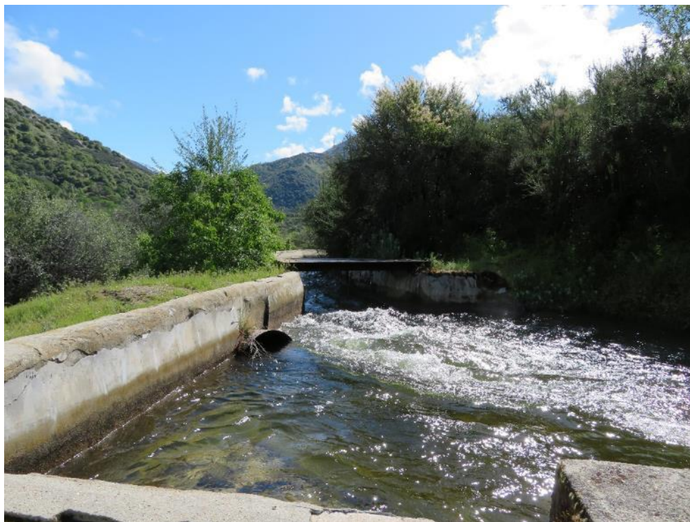
Figure CUL 5-57 Junction of Marble Fork Siphon and Middle Fork Flowline
