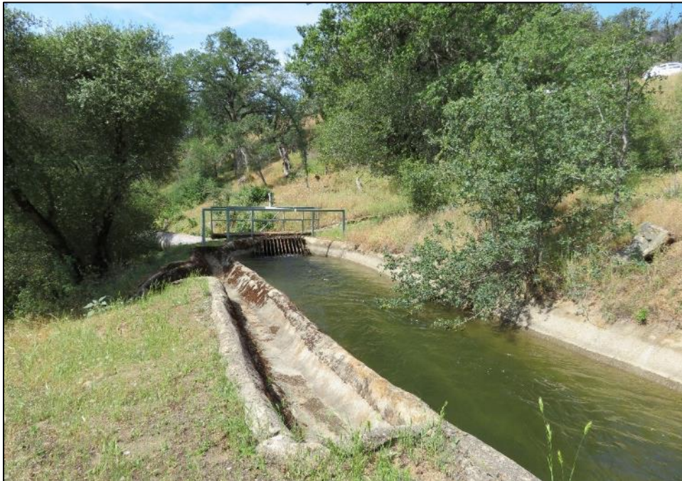
Photograph 9. Spillway and entry trashrack at transition to siphon pipe, camera facing southwest. May 8, 2018.
