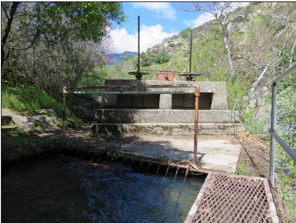
Photograph 5. Middle Fork Diversion trash rack, and slide gates, camera facing west. April 17, 2018.
