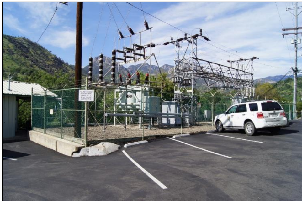
Photograph 7. Kaweah No. 1 Switchyard, camera facing northeast, May 18, 2018.
