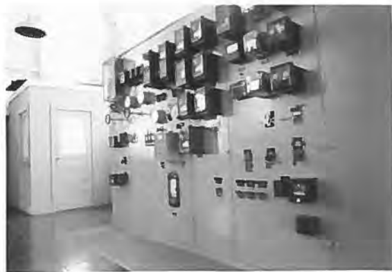
Bldg. 0101, Control Panel Kaweah Powerhouse No. 2 View to NE Roll 1, Frame 27, 6-27-89
