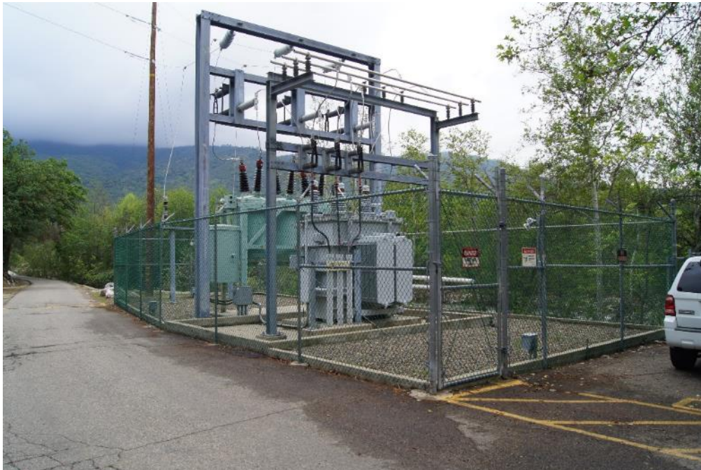
Figure CUL 5-42 Kaweah No. 2 Switchyard, camera facing south
