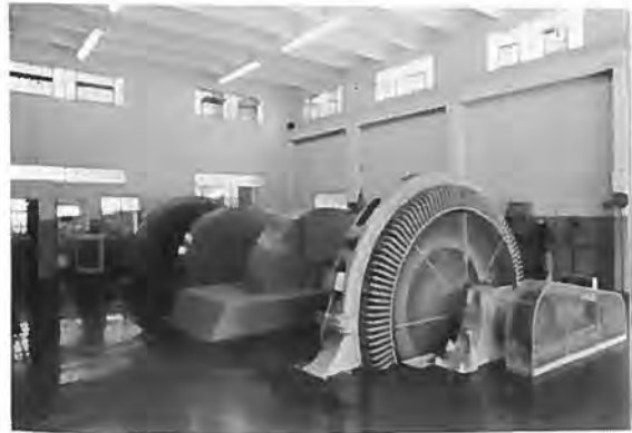
Bldg. 0101, Generator Floor Kaweah Powerhouse No. 3 View to NNW Roll 2, Frame 3, 6-27-89
