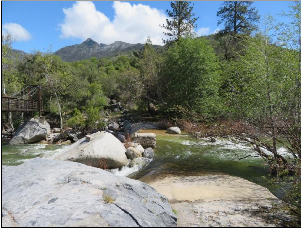
Photograph 8. Siphon covered by concrete at crossing of the Middle Fork of the Kaweah River, camera facing northeast. April 17, 2018.
