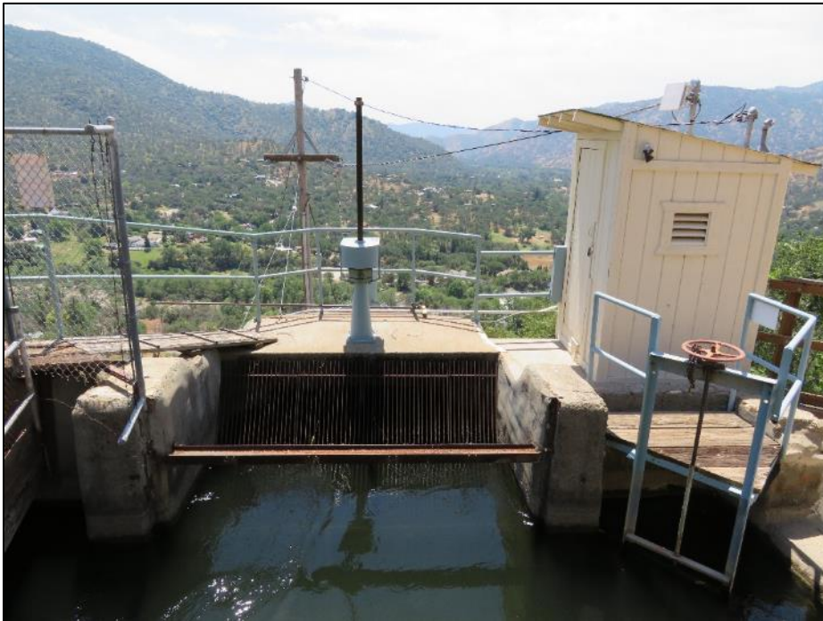
Photograph 3. Trash rack at entry into Kaweah No. 2 Penstock, camera facing southwest. May 8, 2018.
