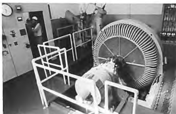
Bldg. 0101, Interior Kaweah Powerhouse No. 1 View to S Roll 1, Frame 3, 6-27-89
