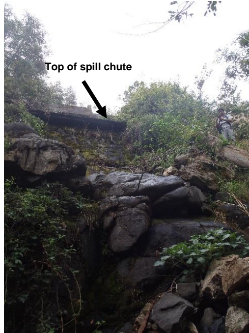
Figure AQ 5-7a. Representative photograph of the upper portion of the drainage chute and natural drainage channel that receives flow from the Kaweah No. 3 Forebay.
