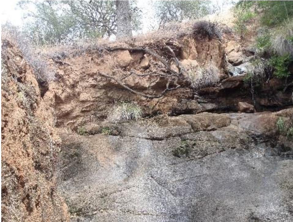
Figure AQ 5-6c. Recent erosion on the side slope of the natural drainage channel which receives flow from the Kaweah No. 2 Forebay.
