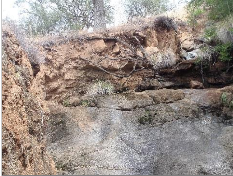
(c) Recent erosion on the side slope of the Kaweah No. 2 natural drainage channel (#1, primary), near the top of the drainage.
