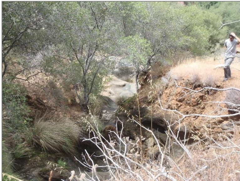
(b) Representative photograph of a down cut section in the Kaweah No. 2 natural drainage channel (#1, primary).
