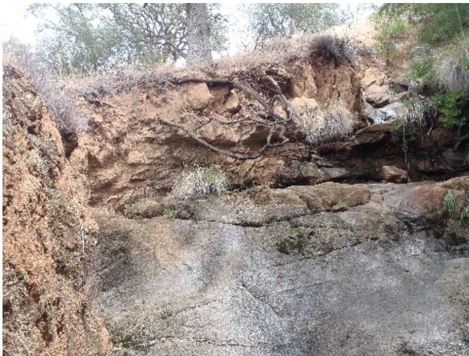
c. Recent erosion on the side slope of the Kaweah No. 2 main spill drainage, near the top of the drainage.
