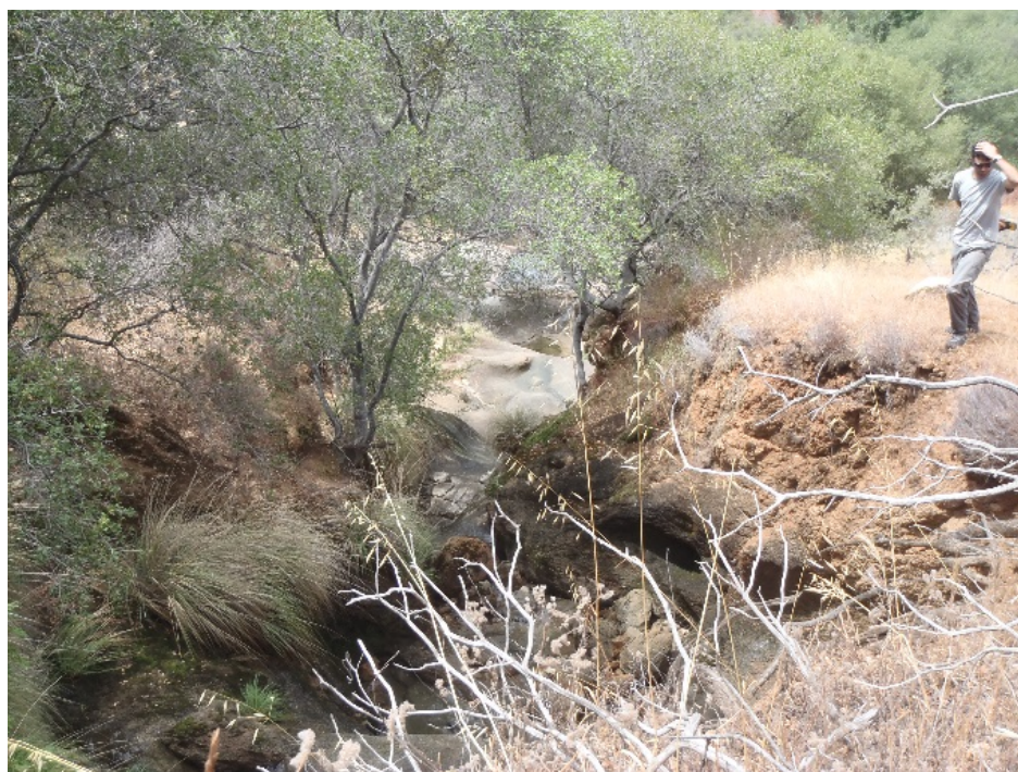
b. Representative photograph of a down cut section in the Kaweah No. 2 main spill drainage.
