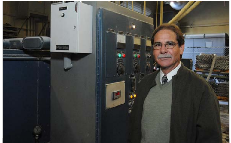
West American Rubber Company President Jim deLeo shows one of the energy management system control boxes (funded by SCE's Technical Assistance and Technology Incentives Program) that allow his company to reduce electricity costs.
