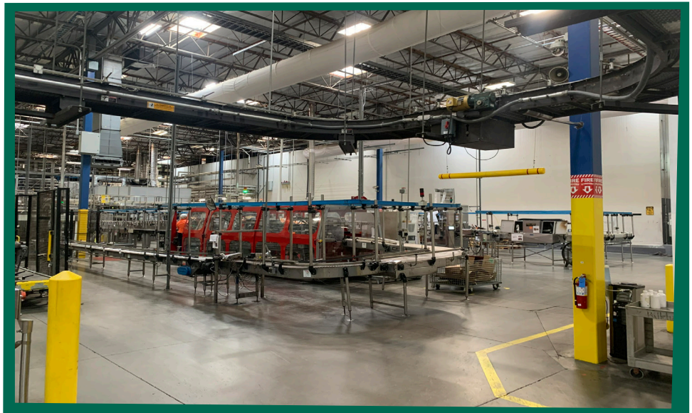
Glanbia saved thousands of dollars after a “treasure hunt” at their Corona facility uncovered 30-40 air leaks by using equipment from SCE's lending library.
