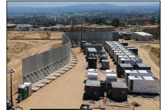
On-site generation and sound walls
